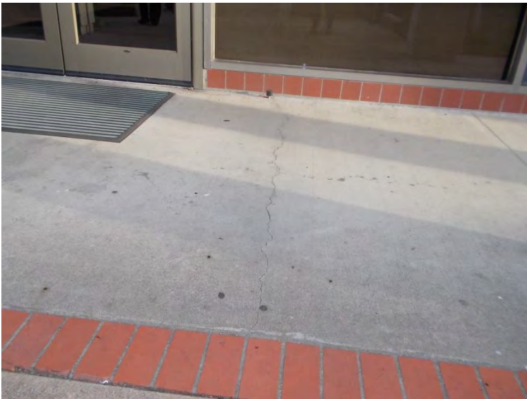
EF4. North side entrance; cracked concrete walkway.
