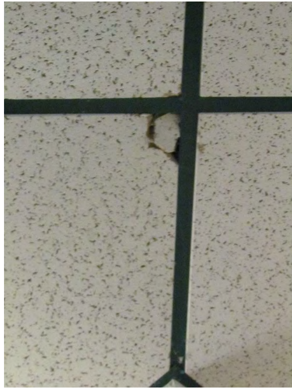
C2. Second floor; ceiling tile damaged.
