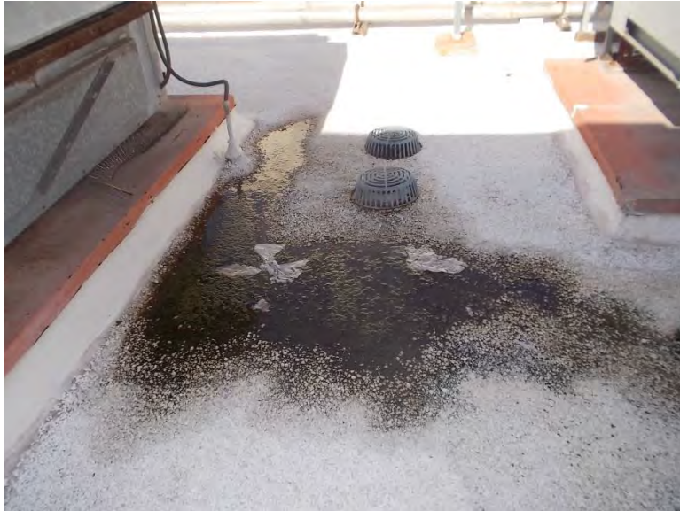
R1. Mechanical roof well with water damage at built up roofing system.
