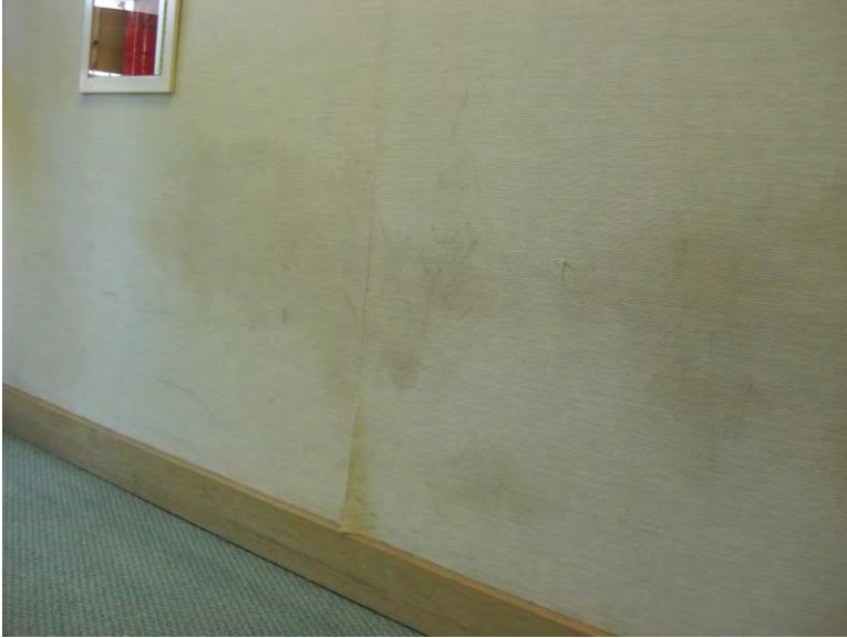
A3. Second floor Corridor 205; fabric covered wainscot stained and damaged.
