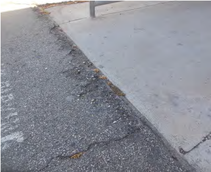
PT6. Landing at ramped walk to Men's restroom; abrupt change in level.
