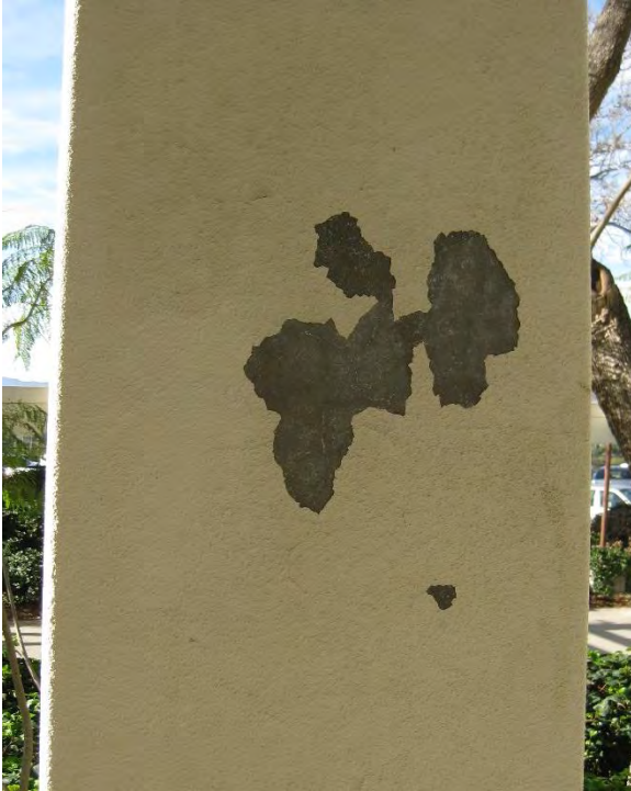
AE1. Exterior columns; peeling plaster paint.
