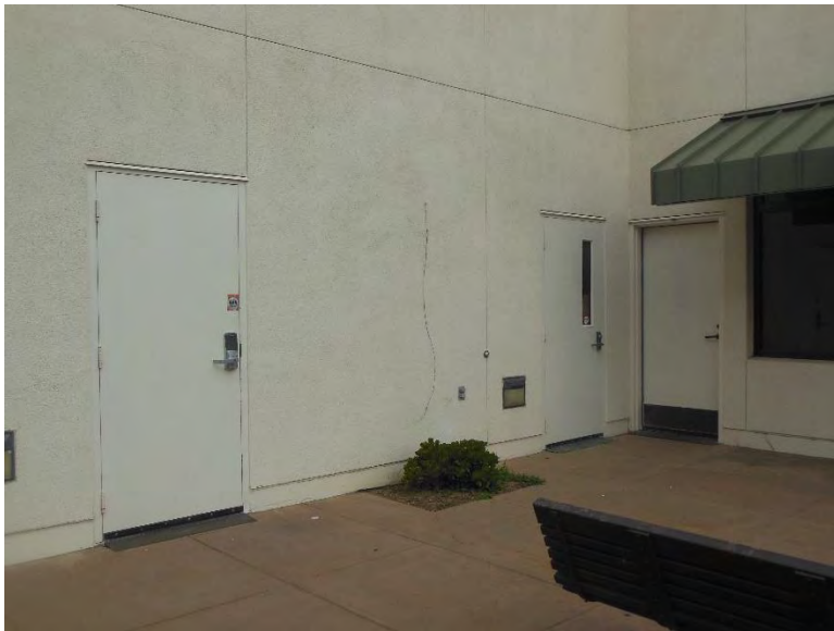
D4. Doors on east side of building; lacking code required wall mounted door identification signage.
