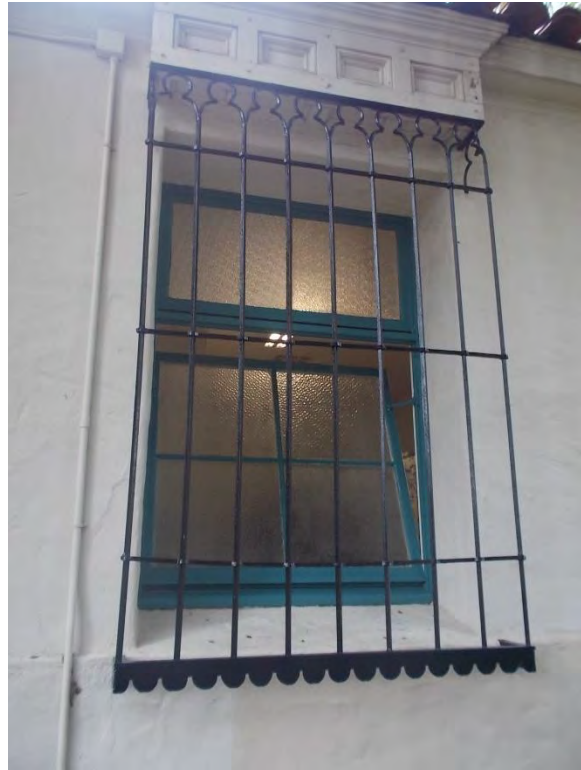
EW2. Women's restroom operable wood window with bars, and newly painted frame.
