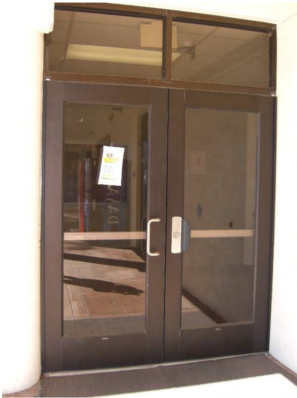
D3. First floor west lower entrance doors; Right hand door abuts the adjacent wall without providing hand clearance to avoid pinching.
