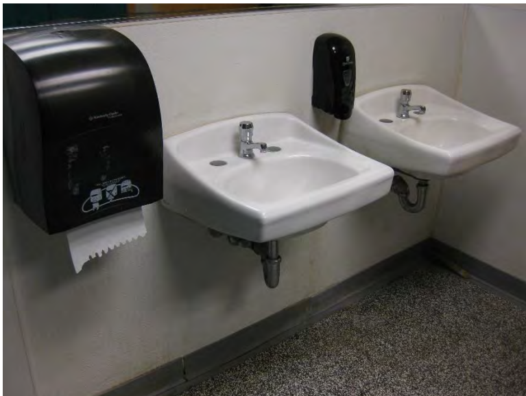
RR2. Sink does not provide paddle faucet fixture handles, knee protection is not provided at under sink plumbing traps.
