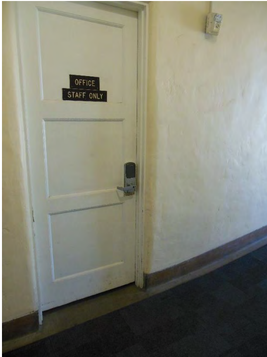
D3. Office 15; interior painted wood door, ADA room ID signage not provided.
