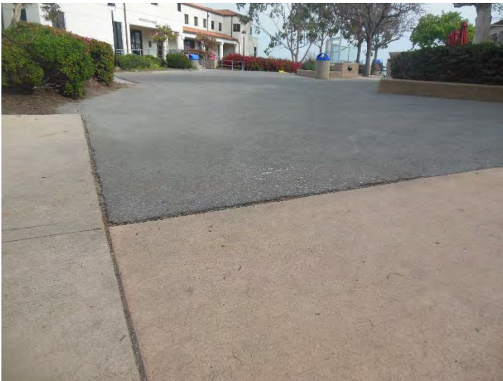
PT9. Northeast exterior walkway; uneven asphalt to concrete transitions. Abrupt change in level and hazardous surface features along path of travel.
