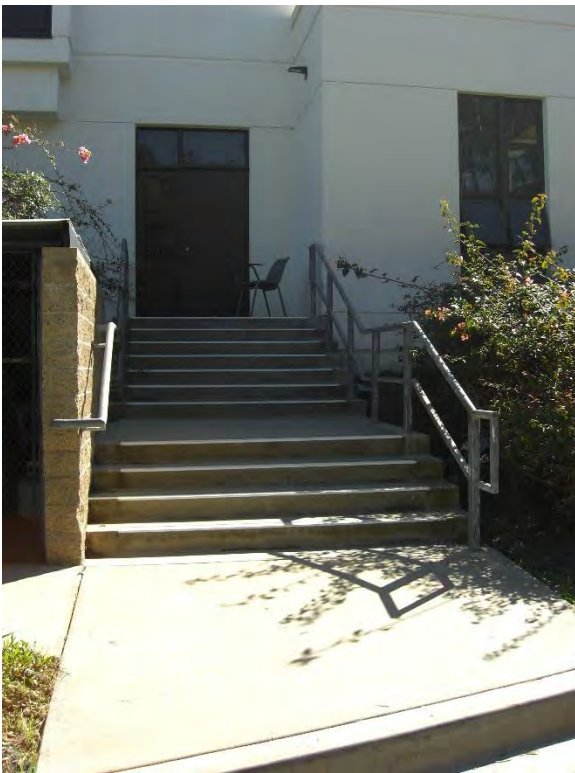
ST2. North exterior stairs with non-compliant and corroded handrails.
