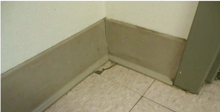
IF5. Corridor 112; original VCT and rubber base in poor condition.
