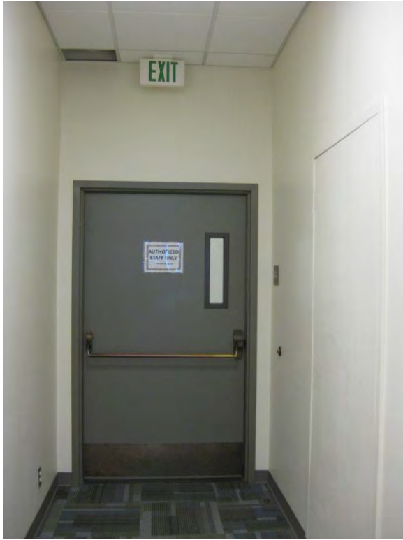
D1. Learning Center area non-compliant exit; side clearance not provided, vision light too high, and exit sign not illuminated.
