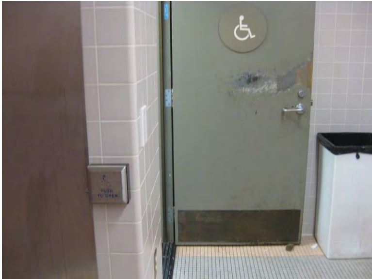
RR1. Women's Lobby restroom. Door finish repair required. Low level access button for electronic door operator is required by code, and ADA door signage is non-compliant.
