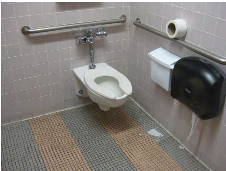
RR2. Women's Lobby Restroom. Dispenser and disposal units protrude into required clear space below handrail.
