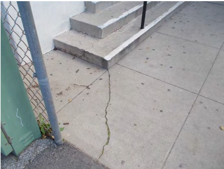
EF2. Exterior sidewalk, west side; cracked and degraded concrete.
