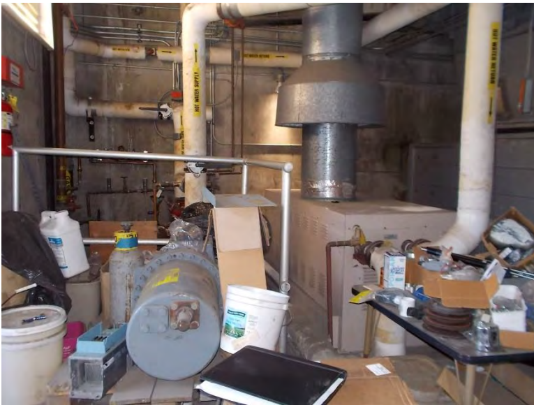
M2. Mechanical equipment blocked by debris.
