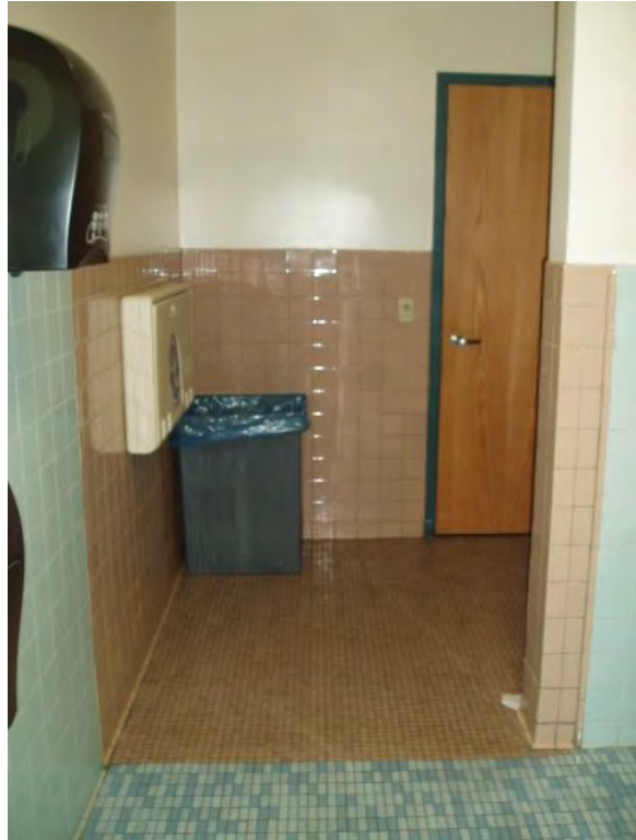
A16. Restroom wall tile mismatched.
