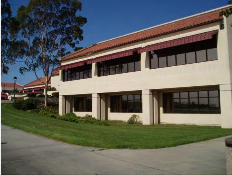
PT1. Non-compliant path at southeast side of building.
