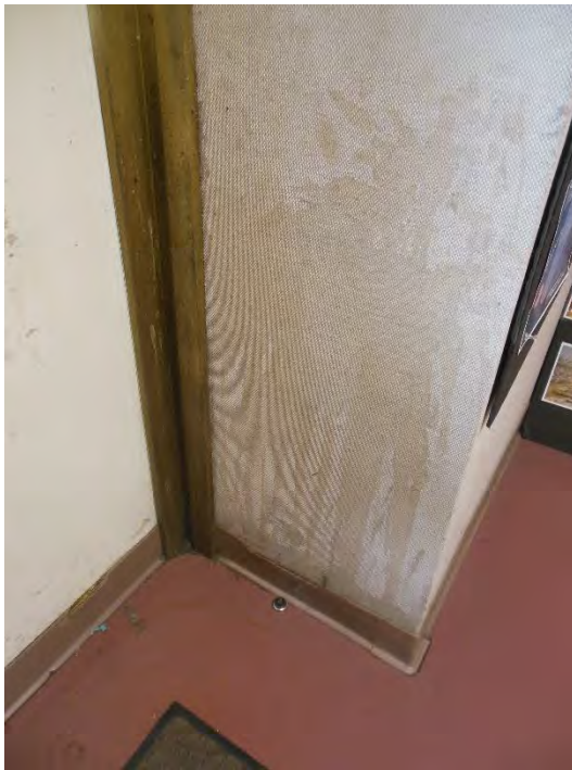
A4. Library vestibule; fabric wallcovering stained.
