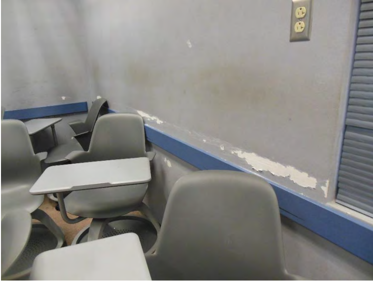
A6. Second floor classroom; paint finish damage from chair backs.
