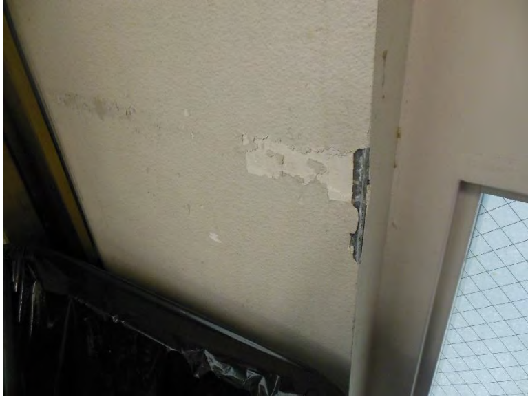
A3. Library vestibule; wall damage.
