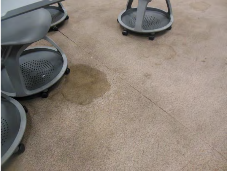
IF4. Second floor classroom, worn and stained carpet, typical.
