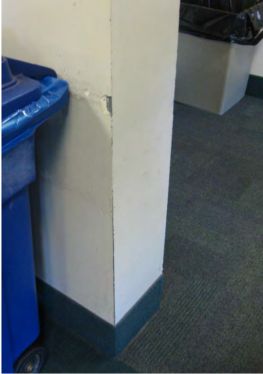
A15. Wing wall damaged corner.
