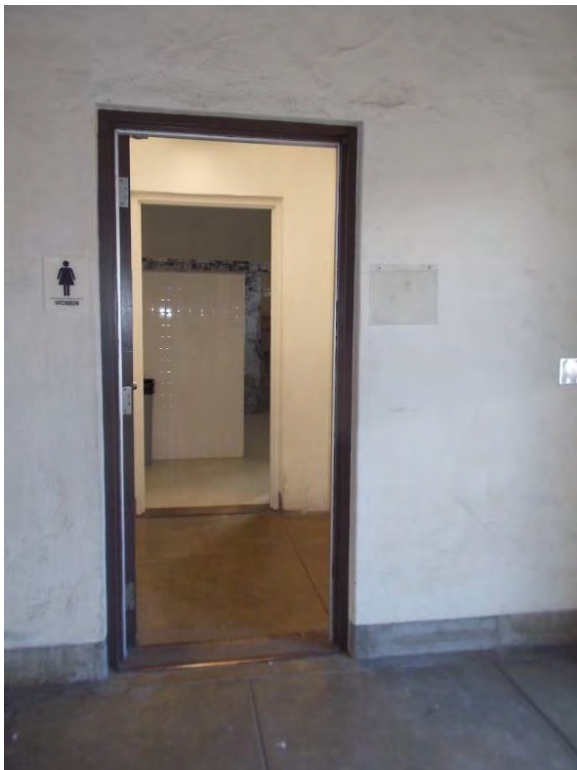
S2. Women's Restroom entrance; room ID signage mounted on wrong side of door
