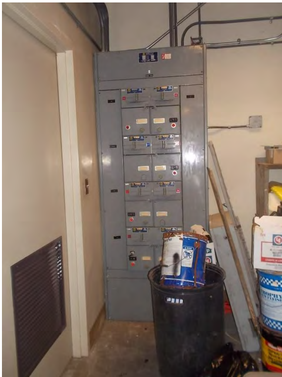
E2. Electrical equipment lacking clear floor space required by code.
