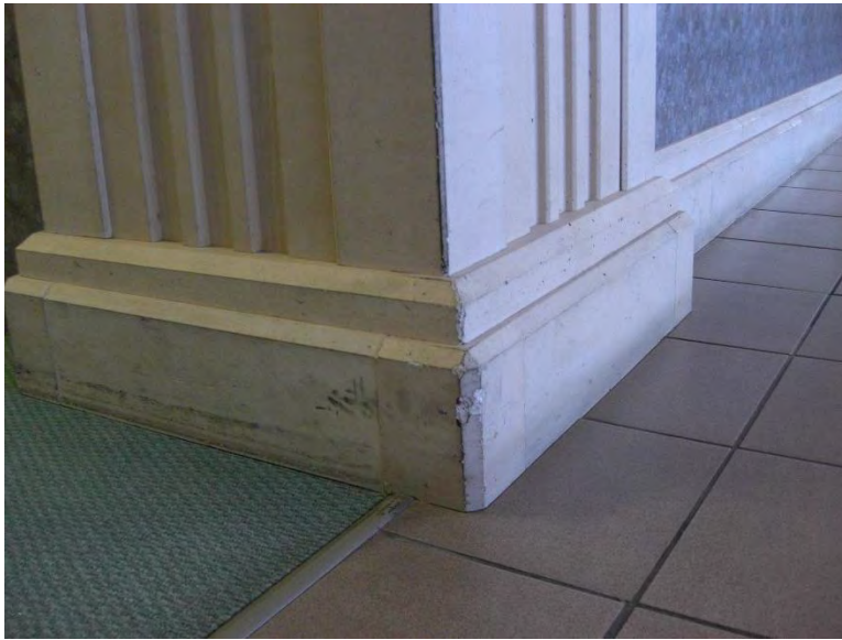
IF1. Second floor reception; wood base damage.
