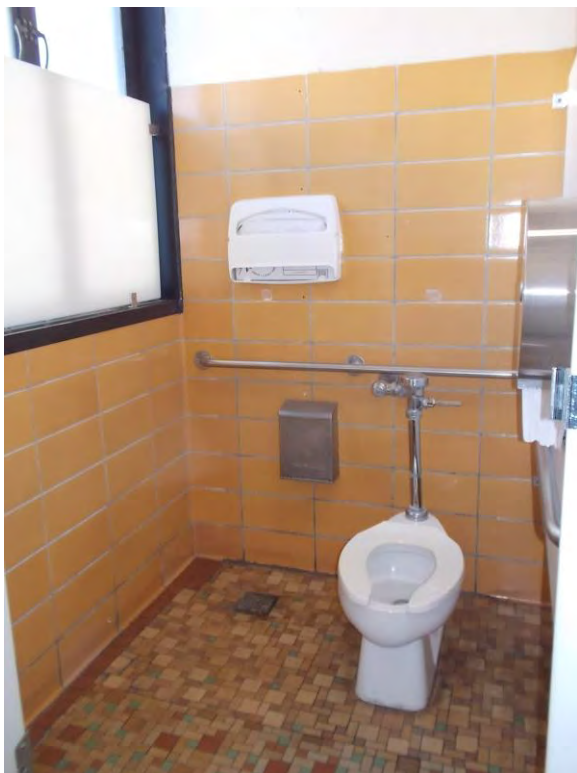
RR2. Womens non-compliant restroom, first floor northwest wing.
