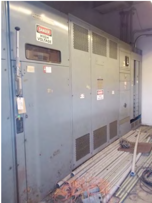
E1. Electrical equipment lacking clear floor space required by code.
