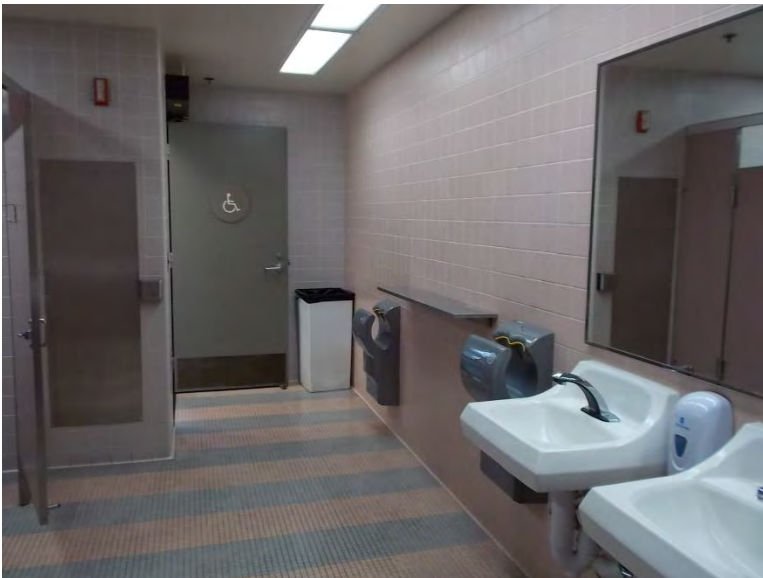
RR2. Womens restroom. Door signage does not meet minimum contrast requirements with adjacent surface.
