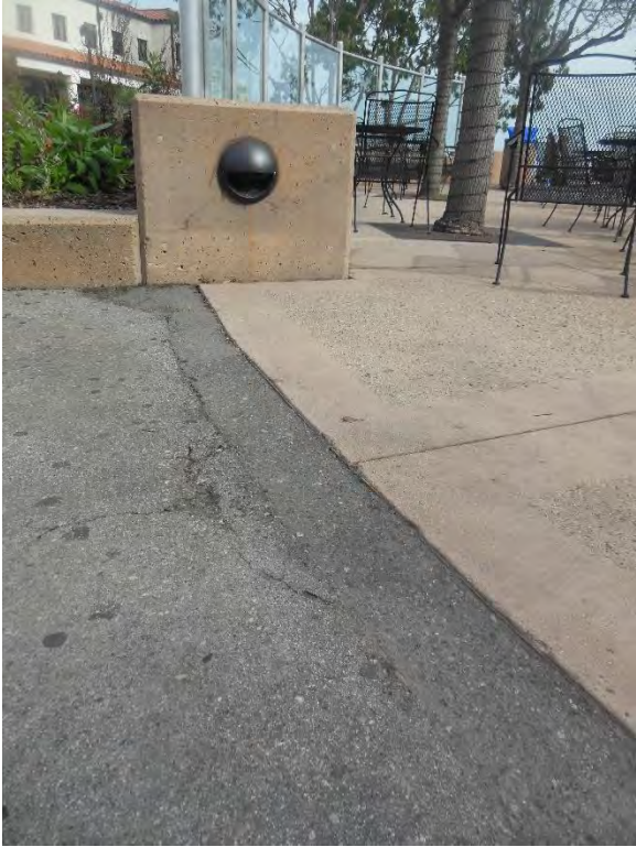
PT10. Outdoor Café pathway material transition; abrupt change in level and hazardous surface features at path of travel.
