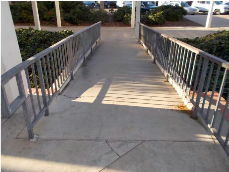
PT1. Exterior north ramp; non-compliant ramp. Handrails heights are too short, gripping surface is too wide, and ramp has excessive running slope. ADA directional signage is not provided.
