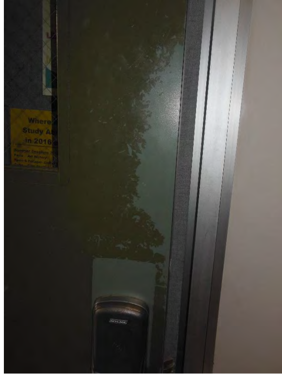
D6. Exterior classroom door; paint finish damaged.
