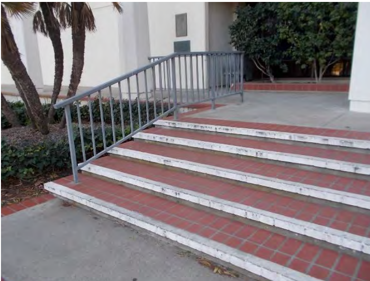
S2. Exterior east stairs; lower handrail extensions are non-existent, gripping surface is too wide, the top and bottom landings have excessive slope and are not level.
