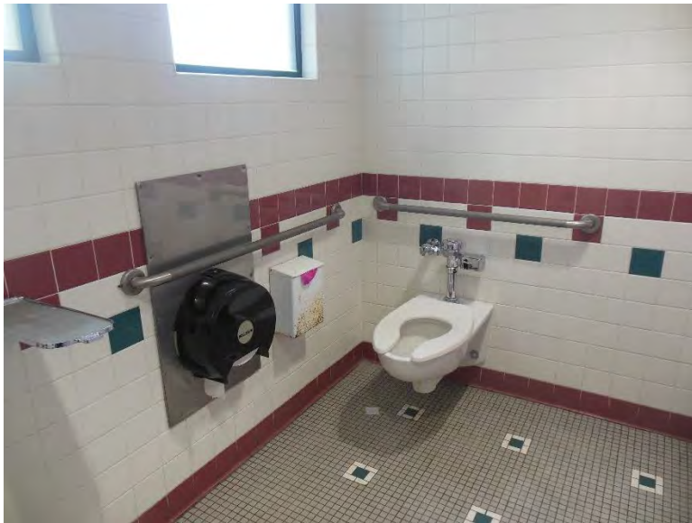
RR4. Cafe restrooms; dispensers may impede forward clear space at accessible stall.
