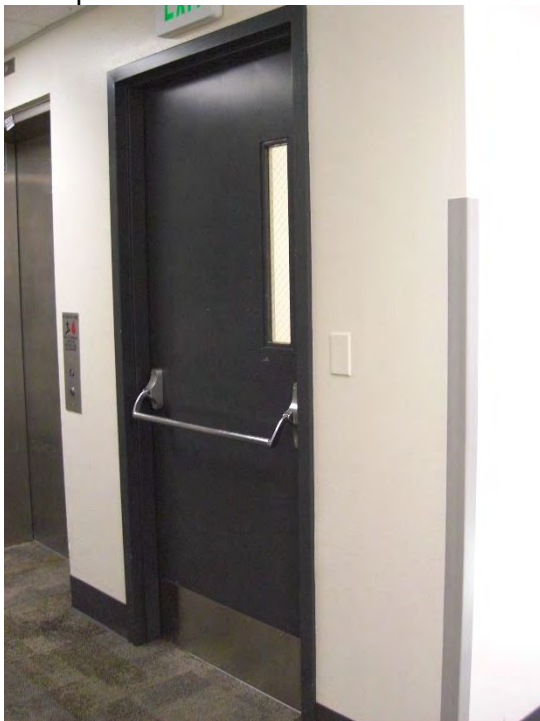
D2. Third floor stairwell door; crossbar style panic hardware does not match other exit doors touchpad style.
