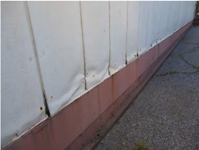
AE4. Portable building, exterior painted siding, damaged.
