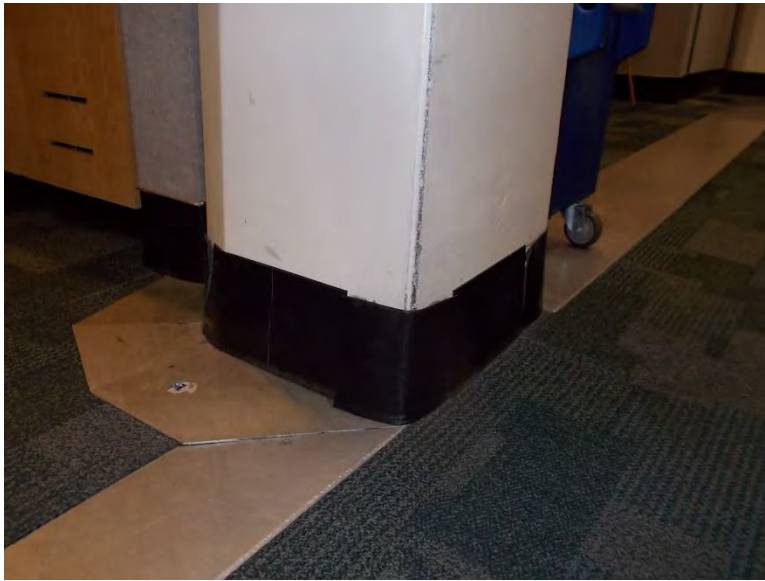
IF1. Second floor Atrium infill space; building expansion joint cover lifted, and rubber base damaged.
