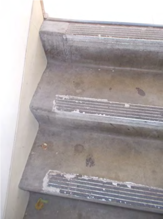
S1. Exterior stairs with non-compliant nosings.
