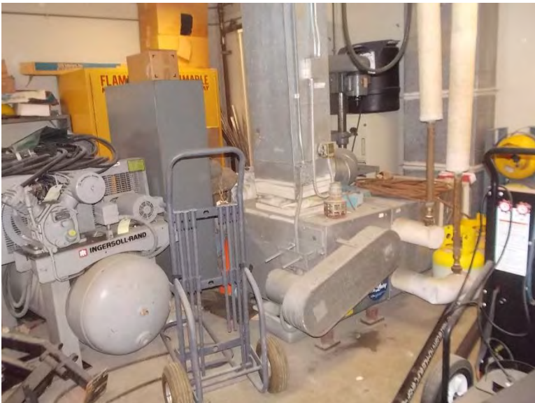
M2. Mechanical equipment lacking clear floor space required by code.
