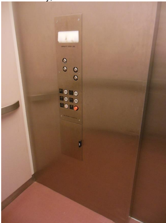
EV2. Elevator interior cab controls.
