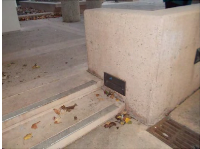
ST2. Exterior south stairs; missing required handrails.
