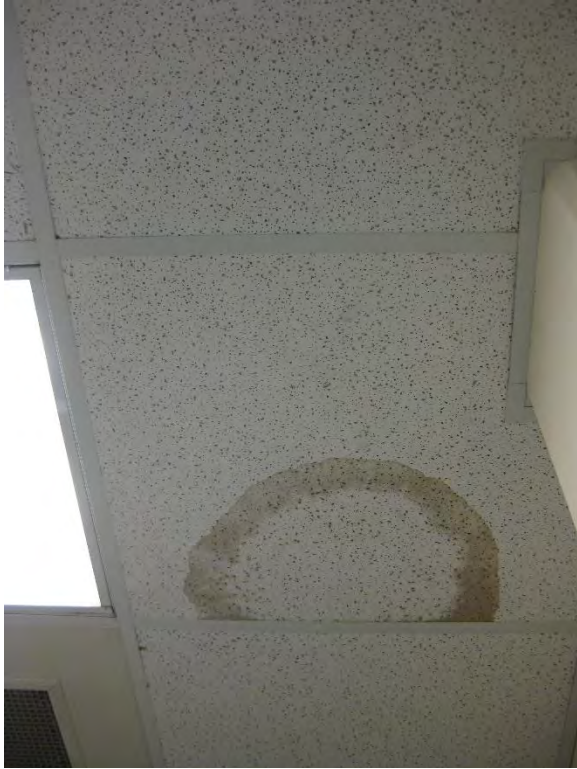
C4. Suspended ceiling tile; stained.
