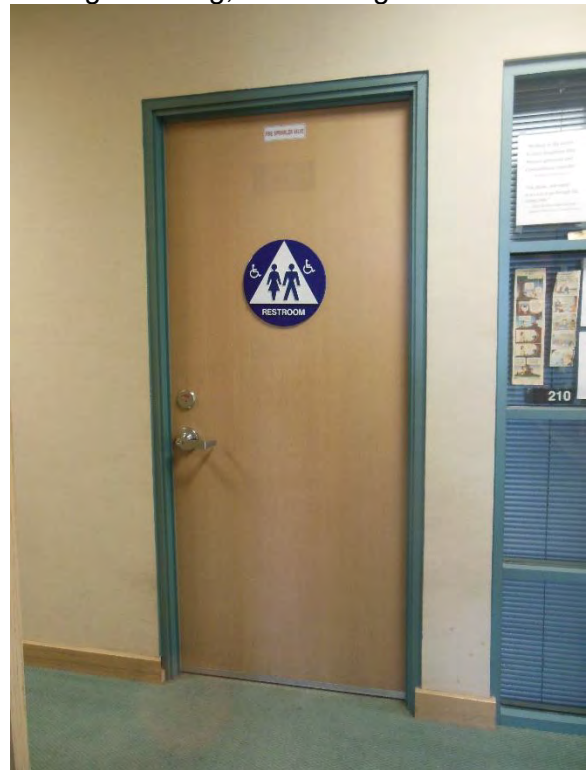
D7. Second floor staff unisex restroom. Missing wall mounted room ID signage.
