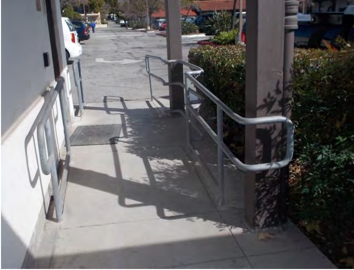
PT5. Ramped walk to Men's restroom; non-compliant handrails.
