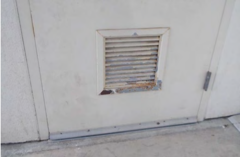
D5. Storage 164 door; damaged louver.
