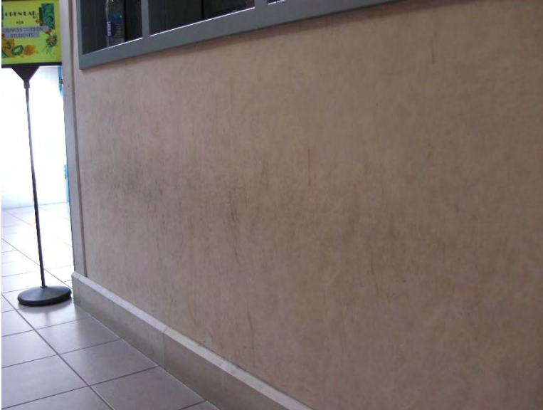
A1. Second floor corridor; veneer plaster wall stained and damaged.
