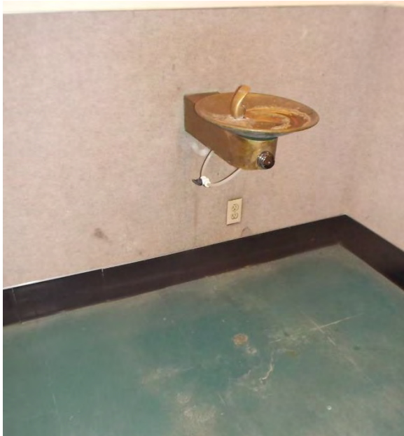
DF1. First floor single drinking fountain; hi-low drinking fountain not provided and flooring damaged.
