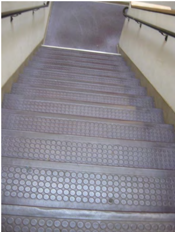
ST2. Library interior stairs; upper and lower visual warning stripes missing at stair nosings. Rubber treads worn and damaged.
