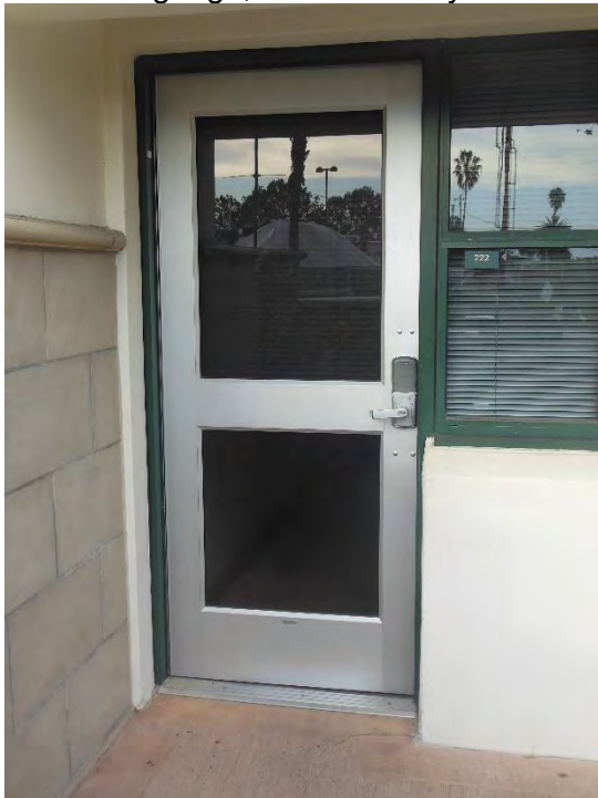
D3. Second floor entry Room 222; lacking wall mounted room ID signage, and pull-side clearance.
