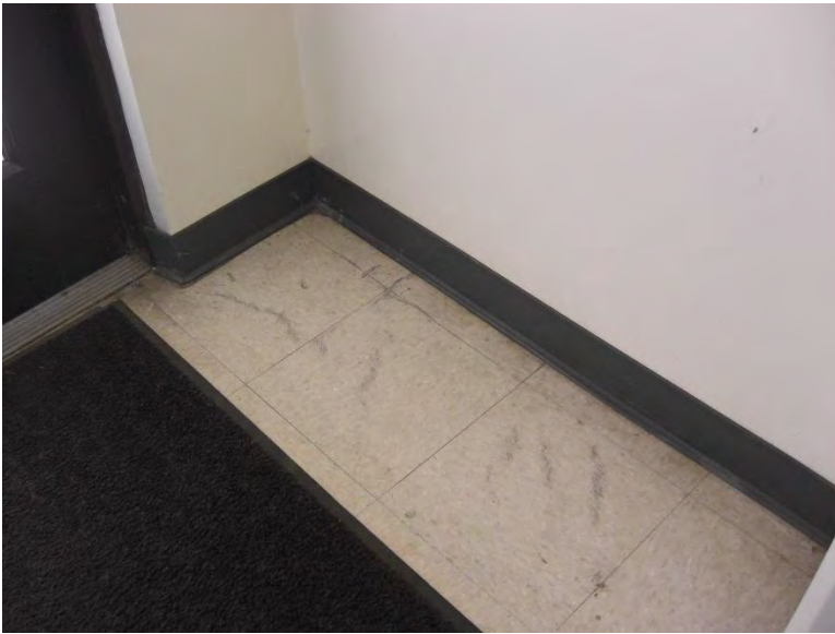
IF1. Second floor entry corridor; cracked and damaged VCT flooring.
