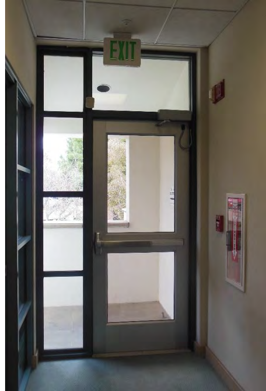
D5. Second floor corridor exit door. Tactile exit sign missing, and exit sign not illuminated.
