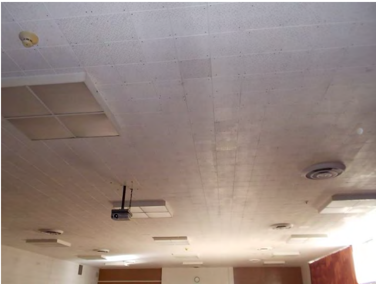
C2. Auditorium; glue on ceiling tiles, screwed into sub-structure.
