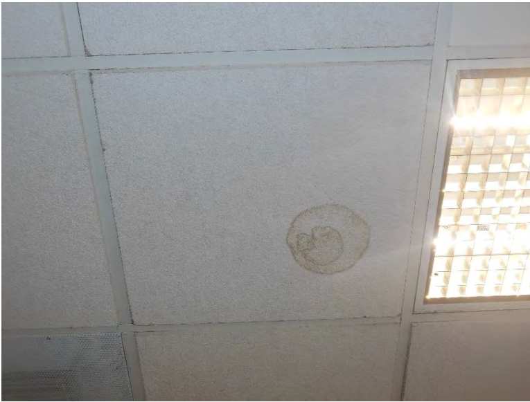
C1. Second floor classroom; stained ceiling tile.
