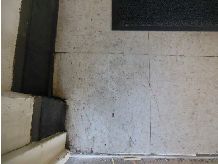
IF3. Office 11 foyer, VCT floor damage.
