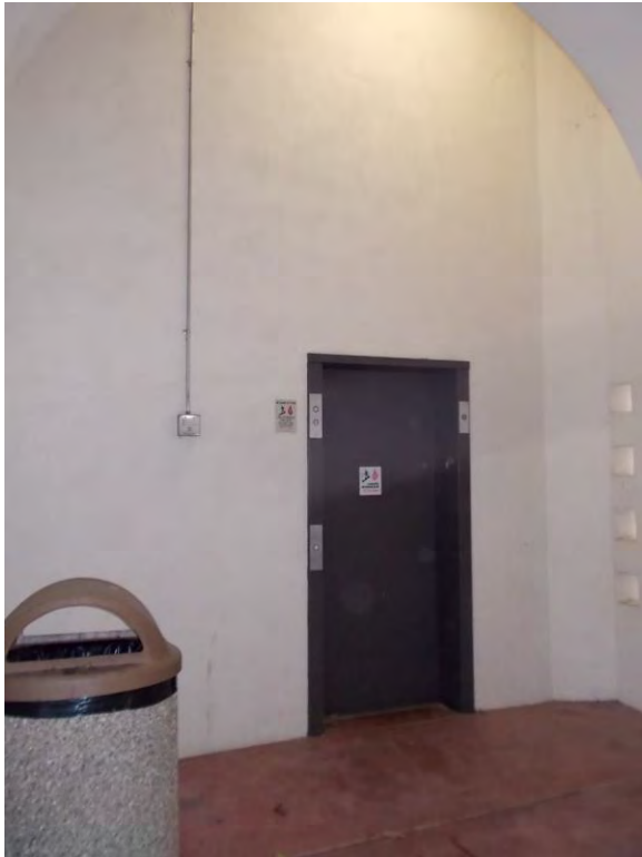
EV1. Elevator as central ADA access.
