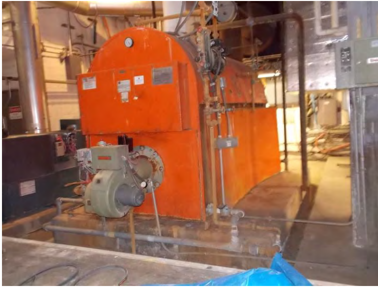
P1. Boiler in basement.
