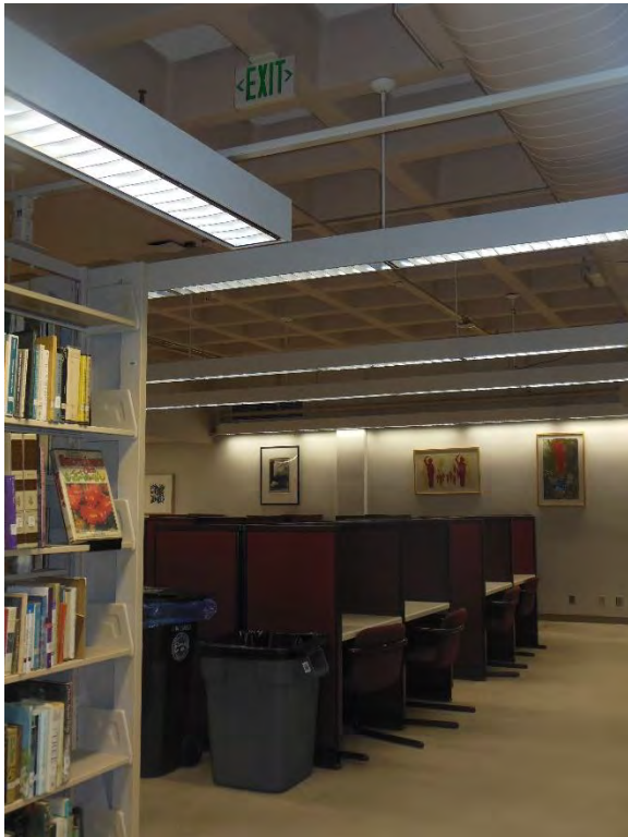
S4. Library, lower level; exit sign not illuminated, and excessively high for visibility.
