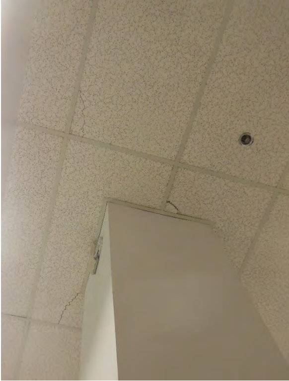
C3. Library upper floor; broken/damaged ceiling tiles.
