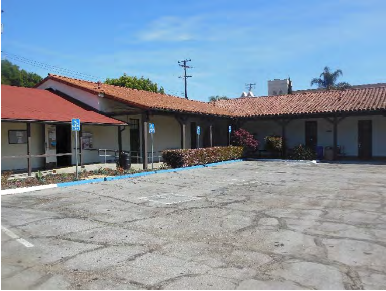
PT9. Accessible stall stripping degraded, layout not-compliant and no safe path from stalls to covered walkway.
