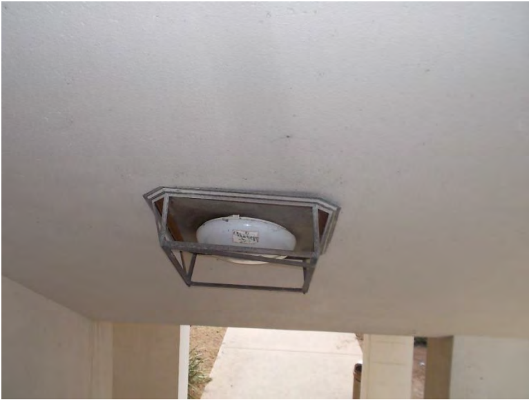
E5. Exterior lighting at northeast stairs.
