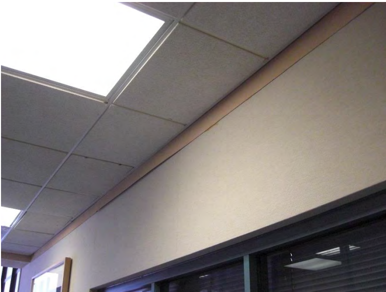
A4. Second floor Corridor 205; head trim piece delaminating from wall.
