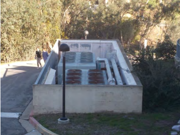
M1. Chiller enclosure. One unit is in use and in good condition.
