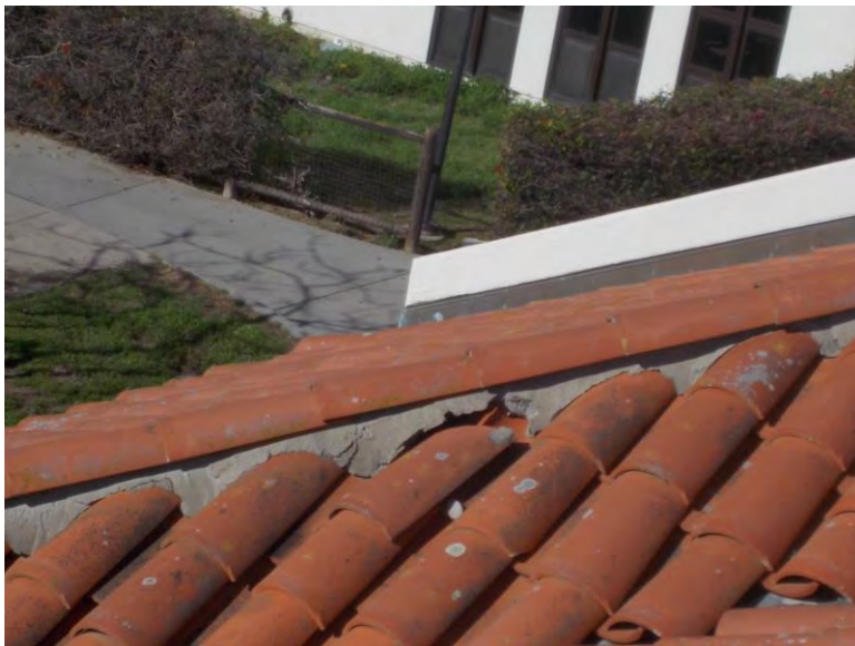
R2. Roof tile mortar damage at ridge, northeast side of roof.
