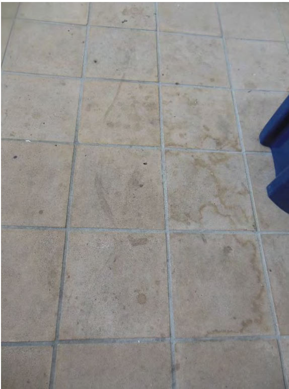
EF4. Third floor exterior walkway; concrete pavers stained.
