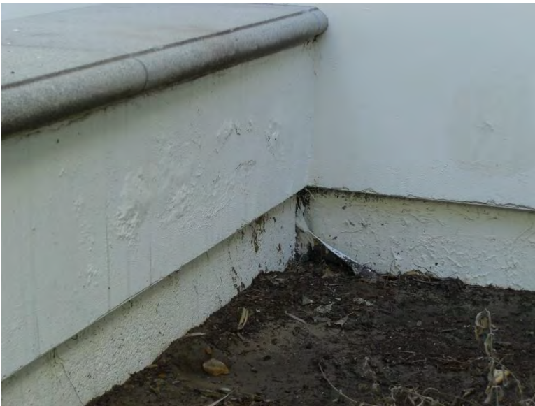
AE2. East exterior wall with bubbling paint.
