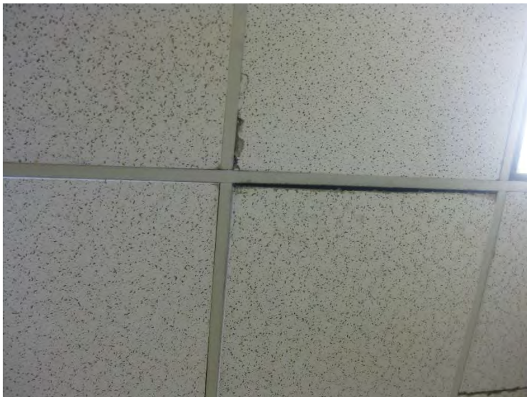
C3. Suspended ceiling tile; damaged.
