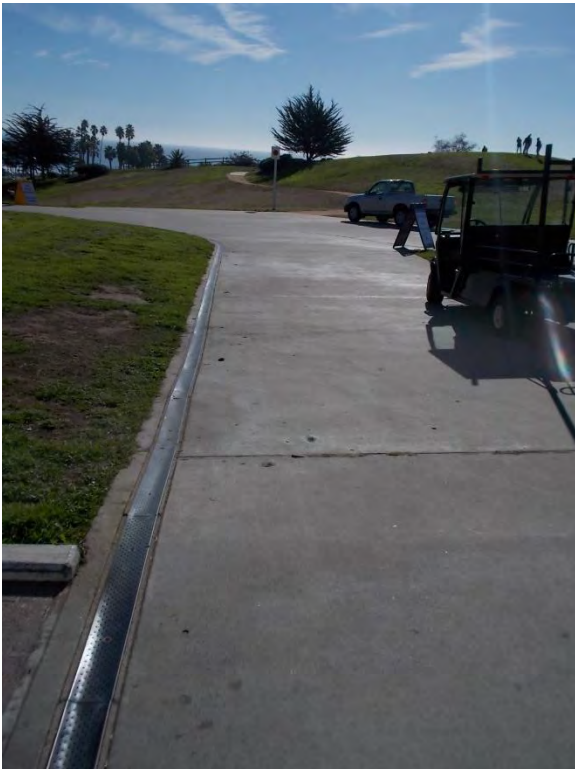
PT2. Non-compliant path at southwest side of building.
