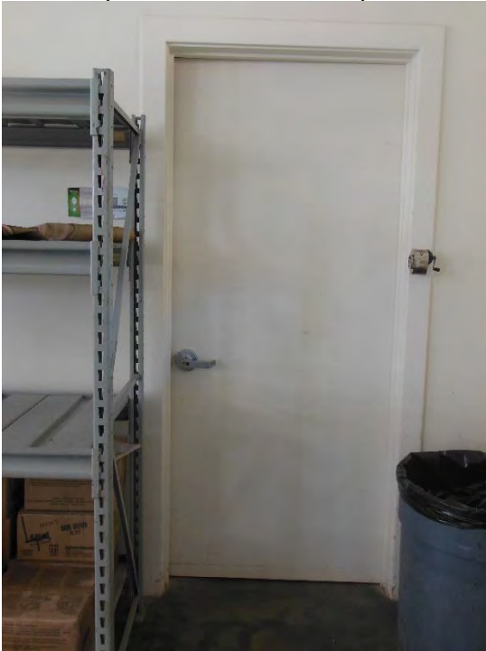
D2. Classroom 22; interior painted wood door, push-side clearance not provided.
