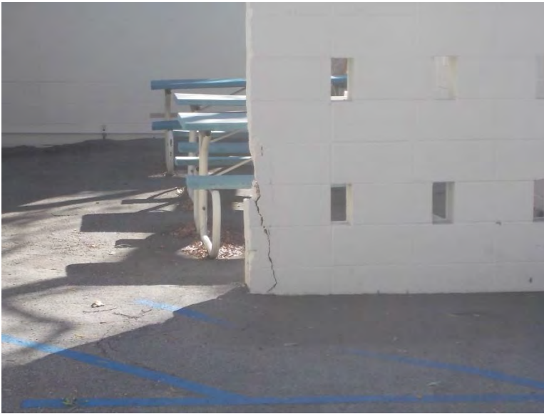
AE1. Exterior patio CMU wall; damaged.
