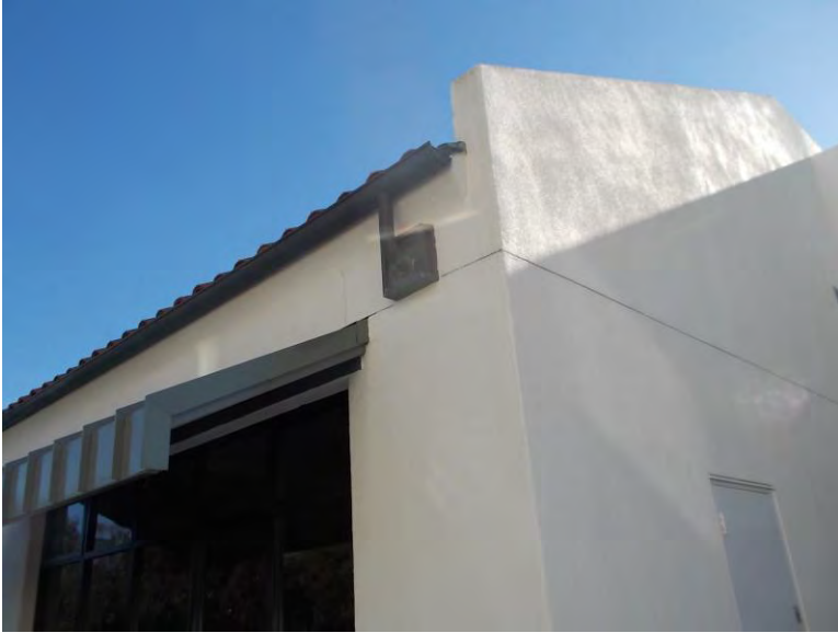
AE1. Exterior walls, minor plaster cracking.
