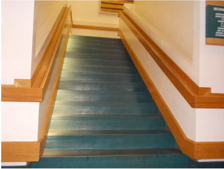
S3. Interior staircase; stair nosings not contrasting, handrails not compliant, and stair signage not provided.
