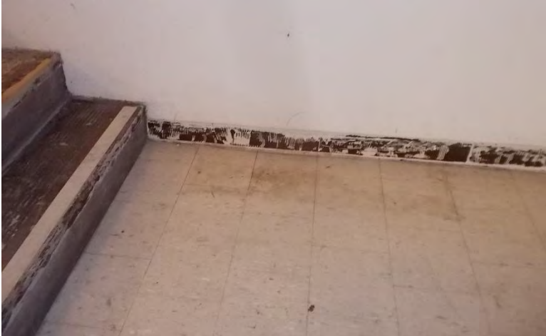
IF3. Basement; base damage at wall and stair riser.
