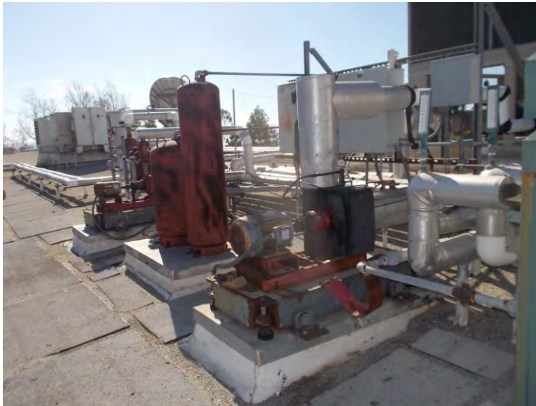
M2. Rooftop mechanical equipment.
