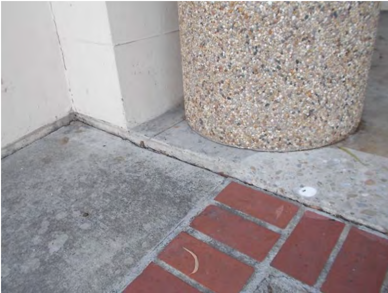
PT2. Non-compliant transition at East ramped entry.
