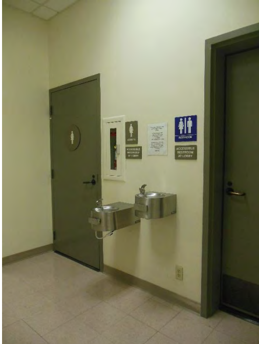
DF3. Corridor 112; non-compliant hi-low drinking fountains.
