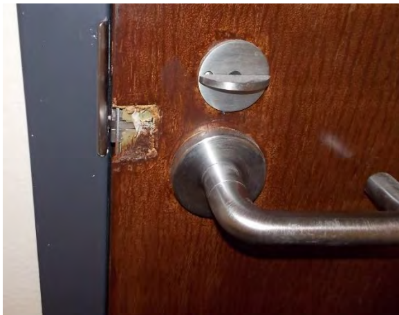
D5. Third floor office door with damage edge at latch.
