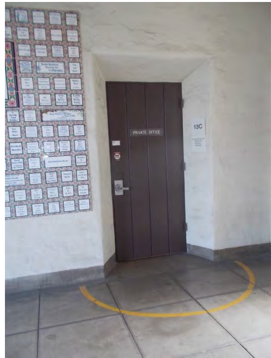
D5. Office 13D door; pull-side clearances not met.
