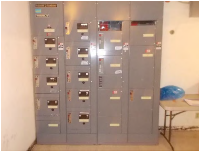
E1. Electrical equipment.
