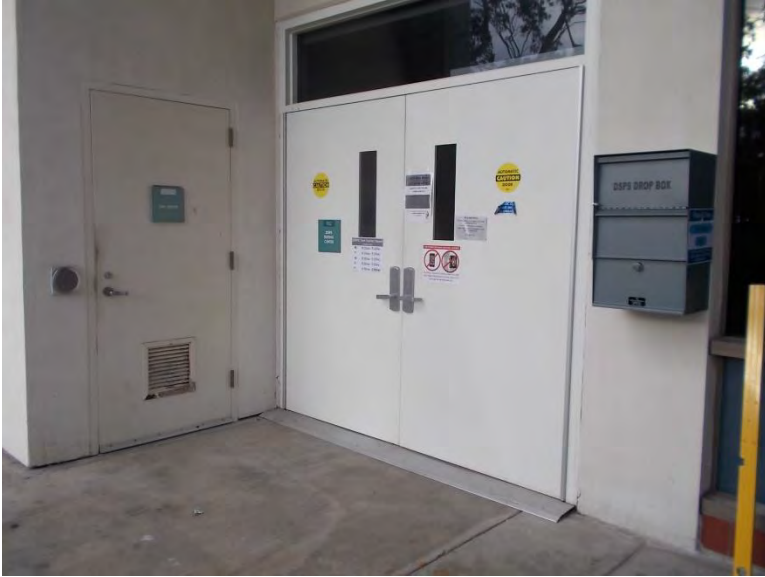
D3. DSPS Testing Lab; non-compliant threshold.
