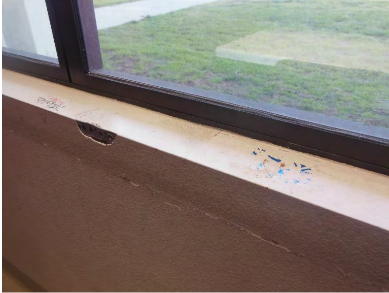
A6. Library south side; lower level window sill vandalism and damage.
