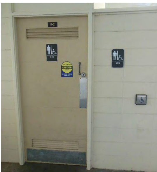
S2. Restroom room identification signs; non-compliant mounting locations.
