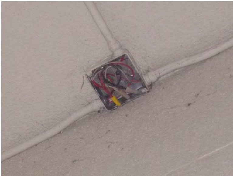
E4. Exposed wiring in j-box.
