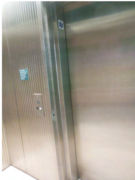
EV2. Braille floor level signs lacking.
