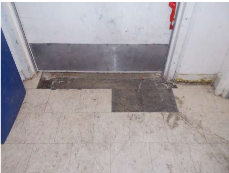
IF5. Basement; 9x9 VAT flooring damage.
