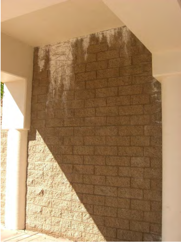
AE3. First floor CMU wall under overhang with efflorescence (white mineral deposits) from water intrusion above.
