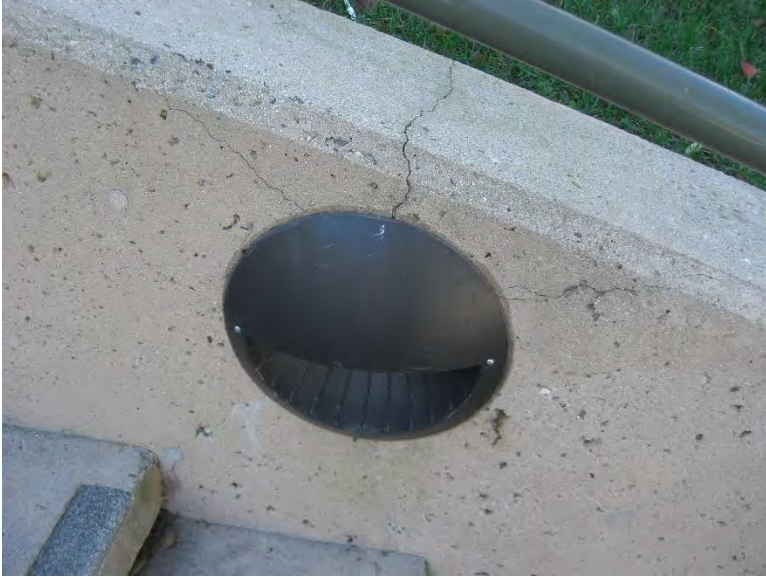
AE5. Cracked concrete wall at exterior stair.
