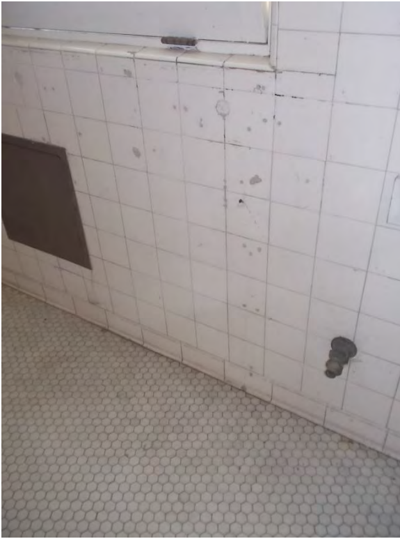
AI1. Women's Restroom, ceramic wall tile damaged.
