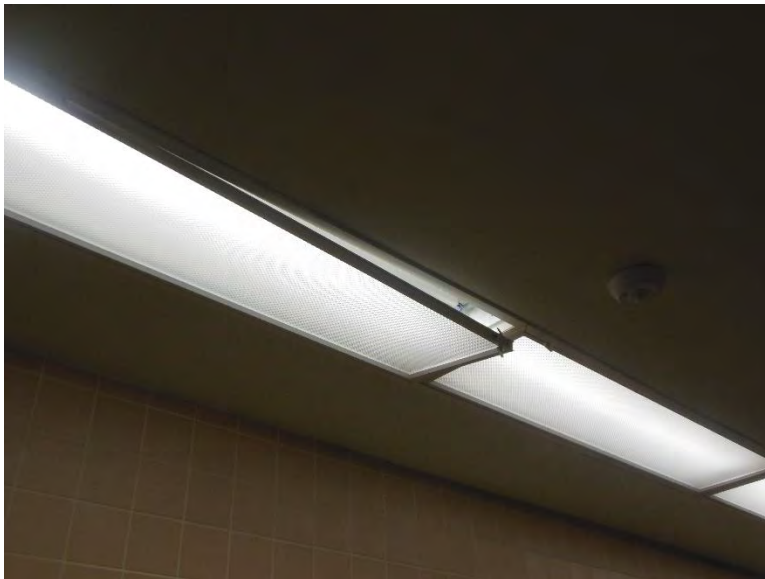
E3. Women's Rstroom 126; lighting fixture lens.
