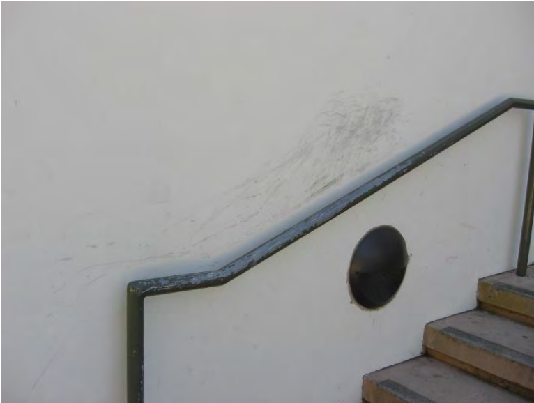
ST6. East side of building; exterior stair handrail finish degraded, and non-compliant height.
