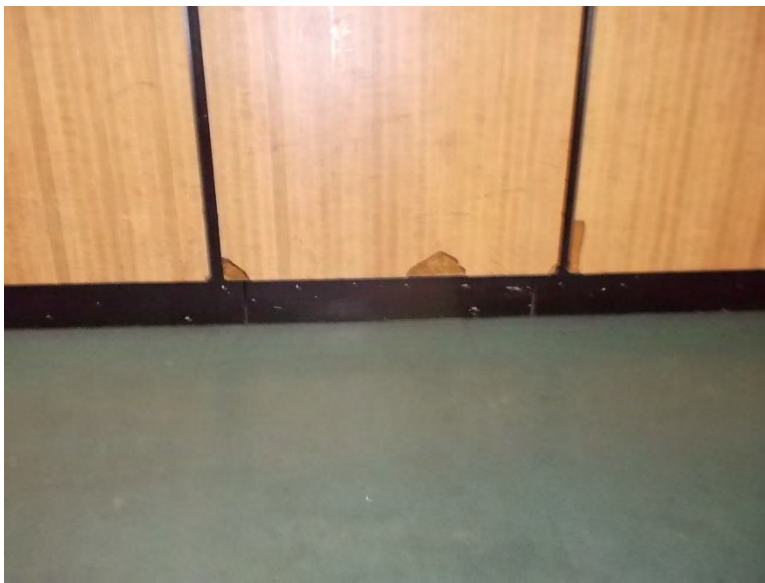
A14. Elevator cab interior; damaged wall panels.
