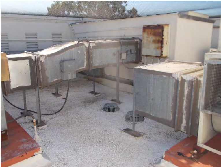
M1. Rooftop mechanical equipment at end of useful life.
