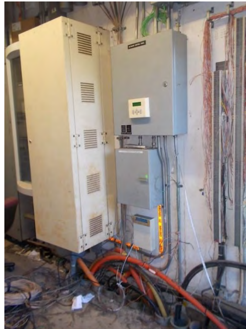
E2. IT and Fire Alarm equipment.
