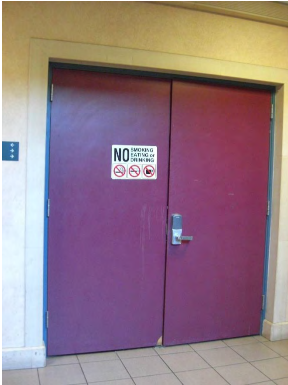
D1. Second floor; damaged and stained plastic laminate faced classroom doors.
