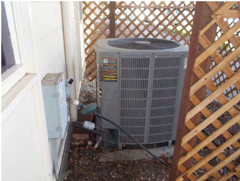
M3. Outside Administration Offices; mini split heat pump system.
