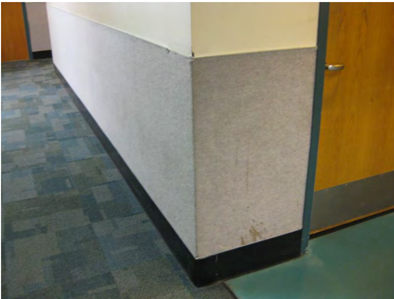
AI2. Second floor corridor; fabric covered wainscot stains and corner damage.
