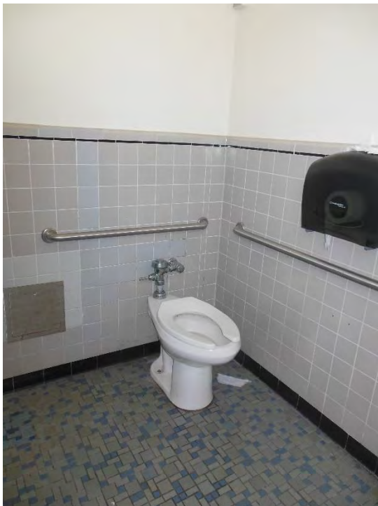
RR4. Men's Restroom; toilet paper dispenser located too high above toilet, and protrudes into clear space above grab bar.
