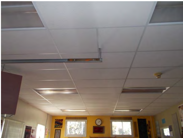
C4. Classroom 32; suspended ceiling system, with recessed lights, typical.
