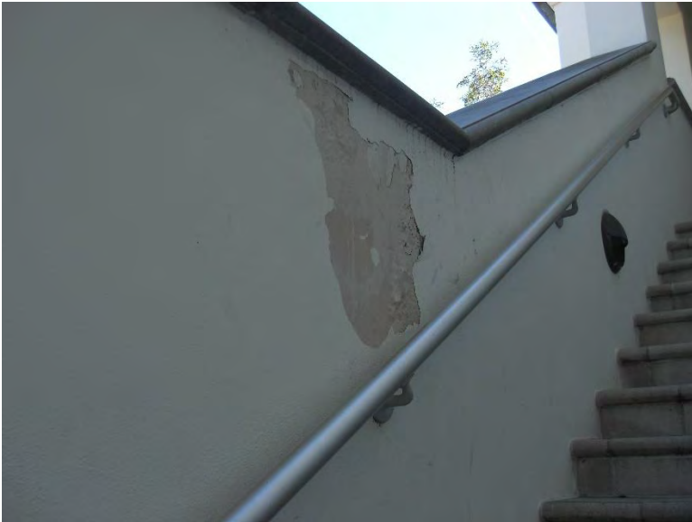
AE4. Exterior east staircase with peeling paint.
