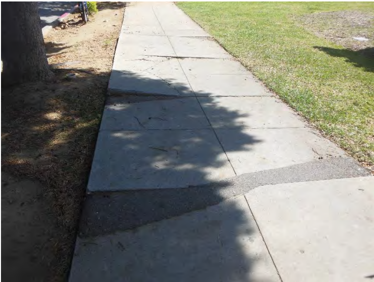
PT10. Public sidewalk at east side of site, near bus stop; abrupt changes in level, and excessive cross slope.
