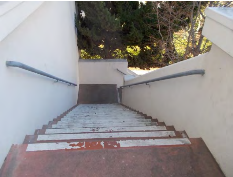
S2. Exterior stairs with non-compliant nosings and handrails.
