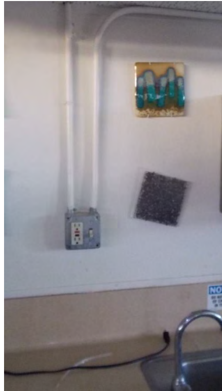
E2. Classroom; exposed conduit and wall mounted duplex outlet.
