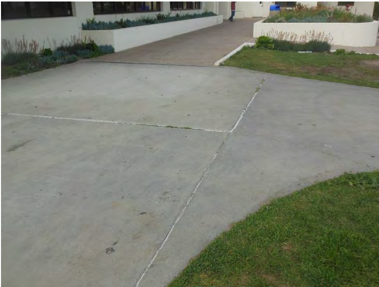
EF2. South side concrete walkway, with excessive longitudinal slope and deteriorated expansion joints.
