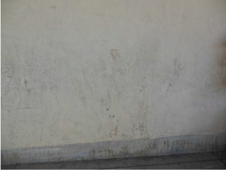
AE3. Permanent building exterior corridor wall; painted plaster damaged.
