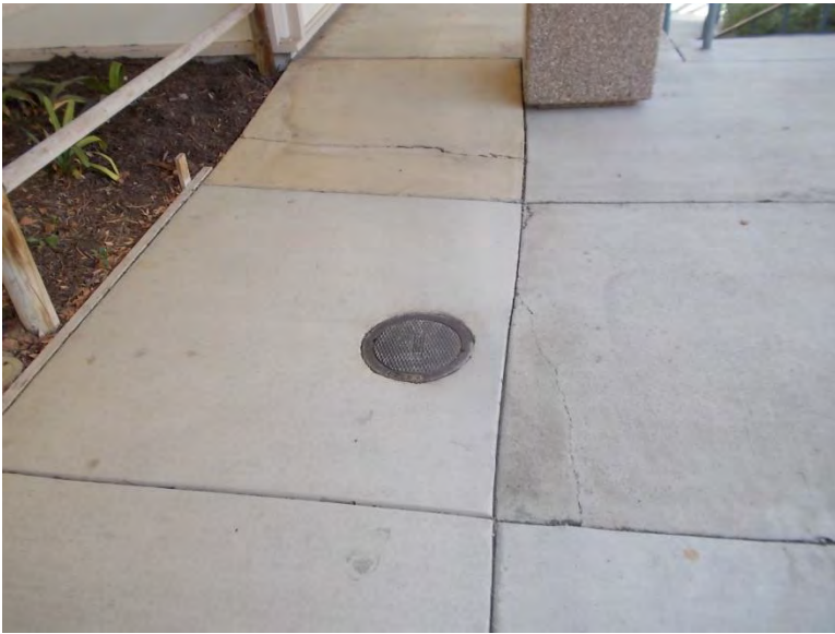
EF1. Exterior corridor walkway; cracked and degraded concrete.
