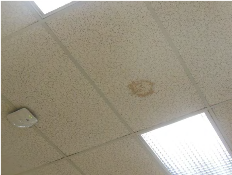
C2. Library second floor; stained ceiling tile.
