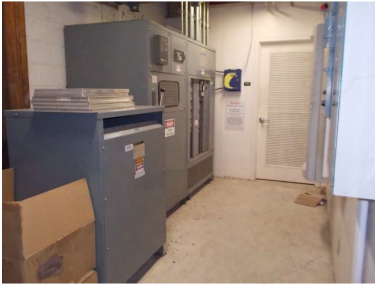
E1. Electrical switchgear.
