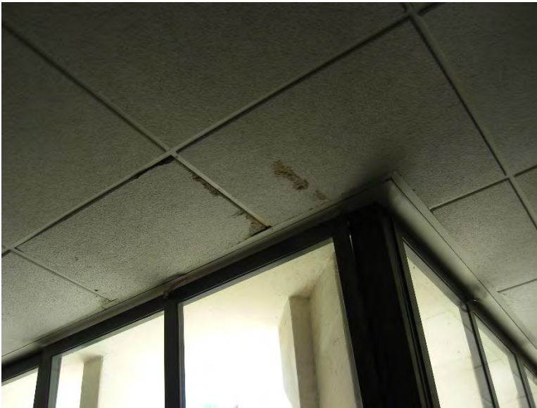
C4. Third floor corridor; damaged ceiling tiles.
