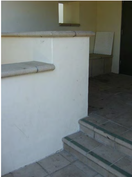
ST1. Exterior north stairs; missing required handrails.
