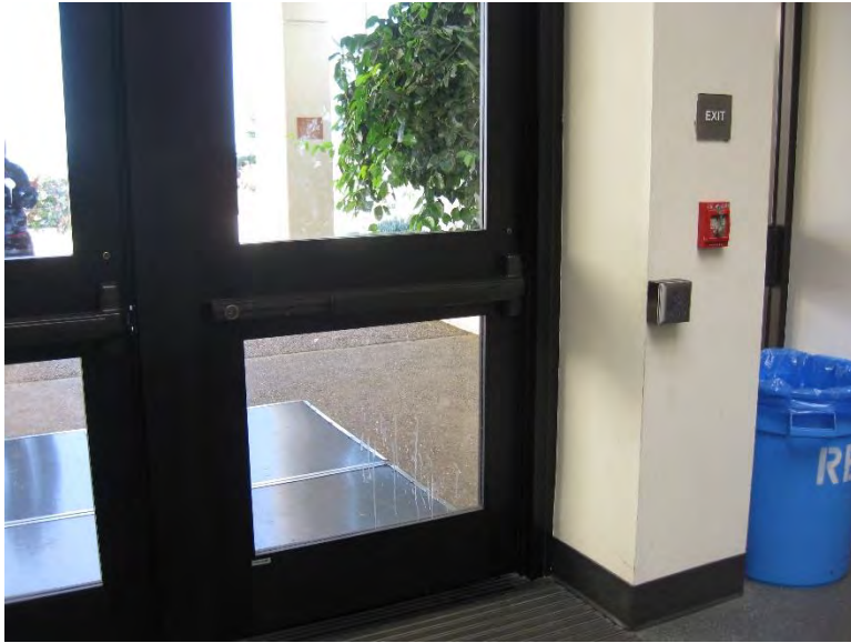
D5. Lobby main doors; non-compliant push-side clearance. Electronic door operator low level access button is required by code.
