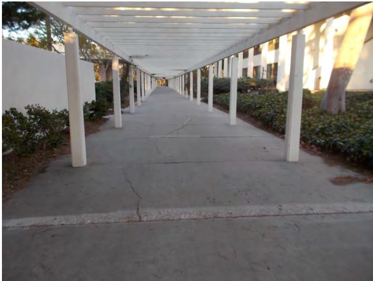
EF2. Exterior walkway; cracked concrete, excessive slopes, and abrupt changes in level. End of walkway terminates into fire truck lane.
