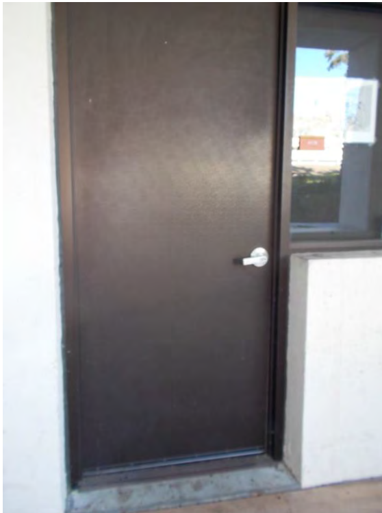
D3. Painted office door at north east side of building, with non-compliant threshold.
