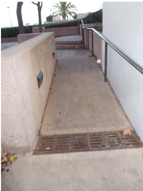
PT7. South side of building, ramp leading to Room 101; One handrail missing, non-compliant height at existing handrail, and drain grate creates abrupt and non-level lower landing.
