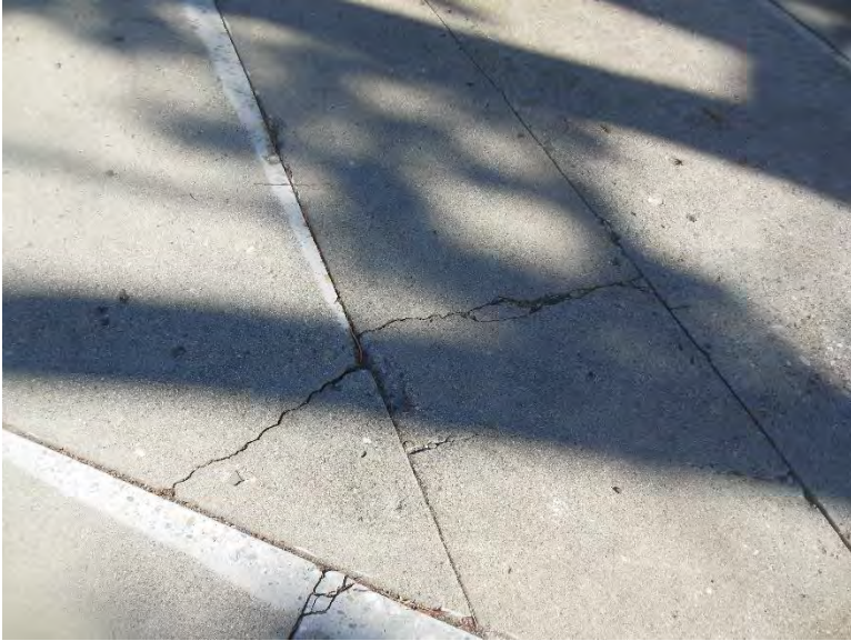
EF3. Exterior corridor walkway; cracked and degraded concrete.
