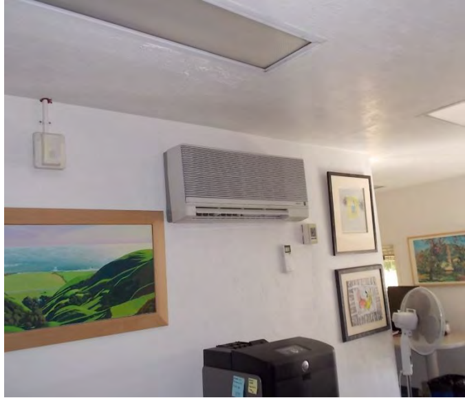
M2. Office 12; wall mounted AC unit.
