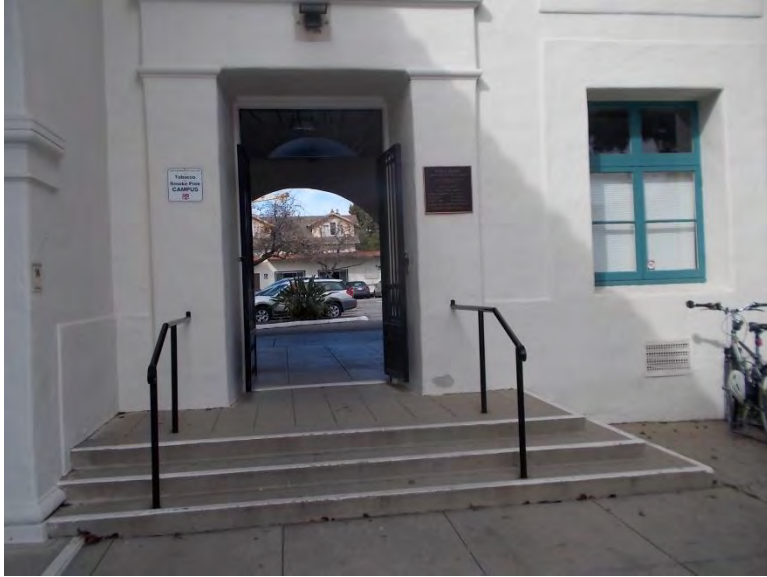
D3. Entrance from south side of site; non-compliant handrail returns.
