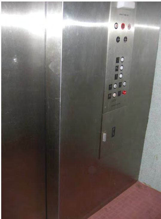
EV3. Elevator car interior.
