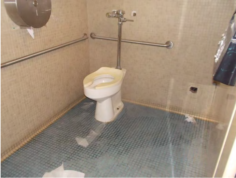
RR3. Men's Restroom accessible stall; ceramic wall finishes have holes and dispenser mounting location interferes with the required clear space above side handrail.
