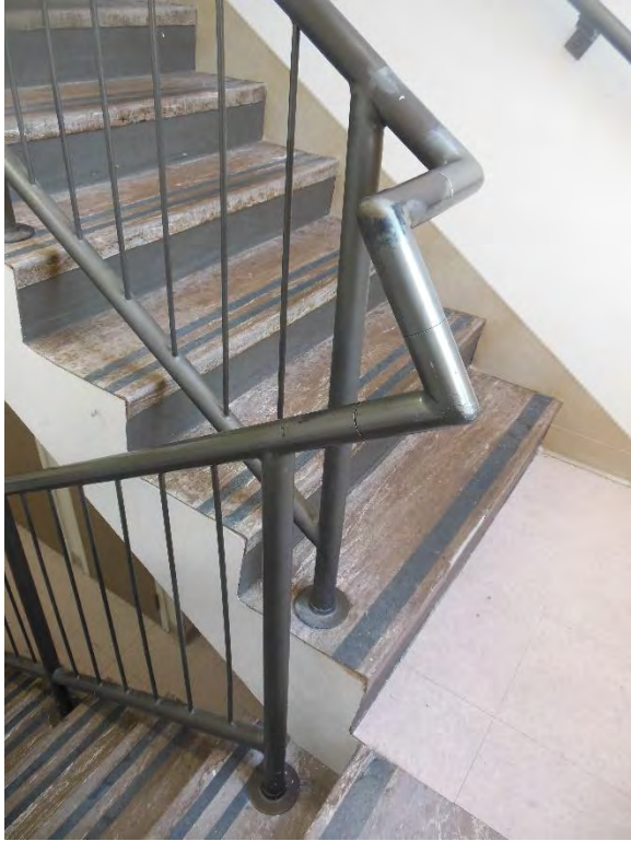
ST3. Stairwell 136; non-compliant handrail heights and returns.
