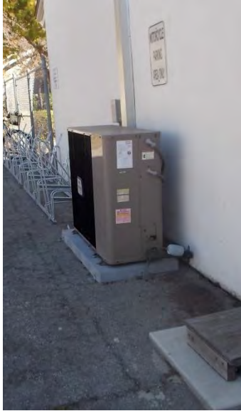
M1. Outside Room 1; mini-split heat pump system.
