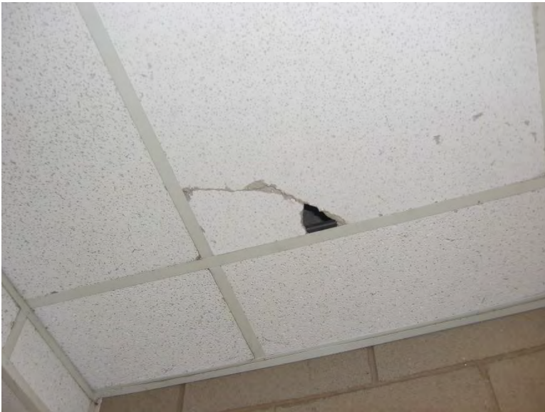
C2. First floor corridor ceiling tile; damaged.
