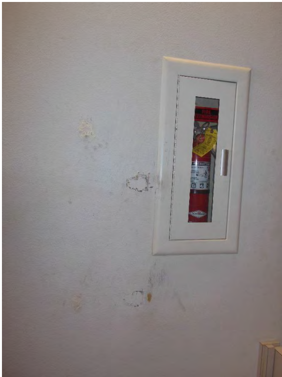
A7. Library lower level; wall damage.
