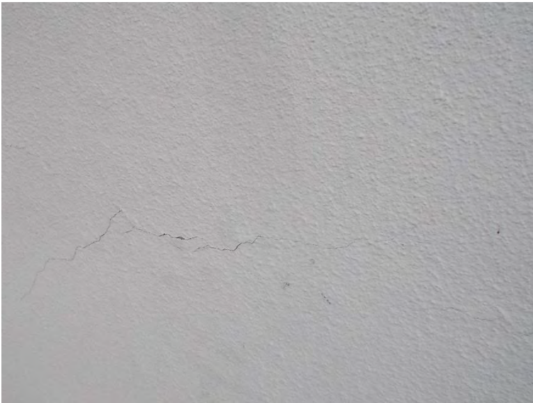
AE4. Exterior wall; cracked plaster finish.
