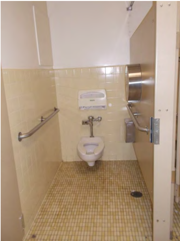
RR4. Women's Restroom ambulatory stall; wall finishes have holes and dispenser mounting location interferes with the required clear space above side handrail.
