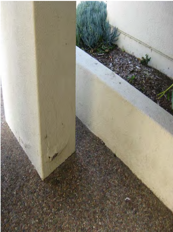
AE2. Cracked and bubbling plaster at south entry column.
