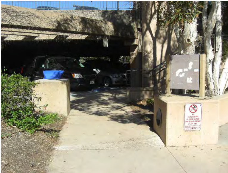
PT1. Paved surface from the IDC building to the accessible parking stalls is uneven and degraded. Path of travel sign is missing.
