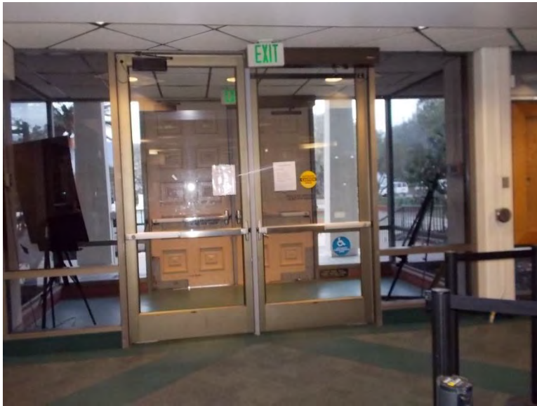
D1. First floor north east exit; electronic door operator low level access button required by code is not installed, and tactile exit signage not provided.
