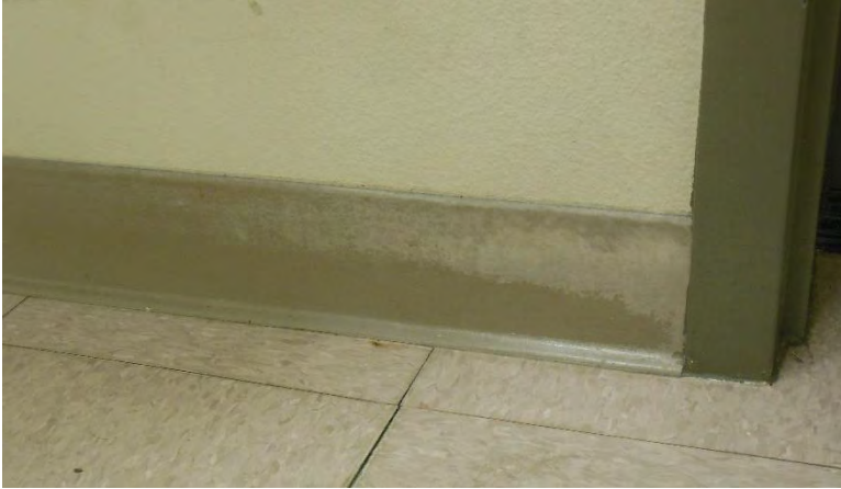
IF4. Corridor 112; original VCT and rubber base in poor condition.
