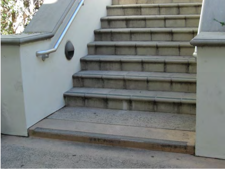
ST5. East exterior stairs with non-compliant landing length.
