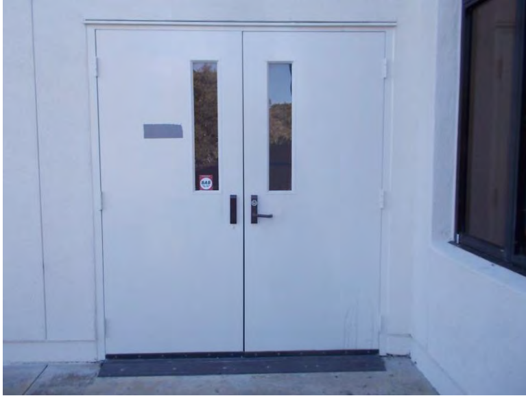
D3. Doors to stairs, at lower level; lacking code required wall mounted door identification signage.
