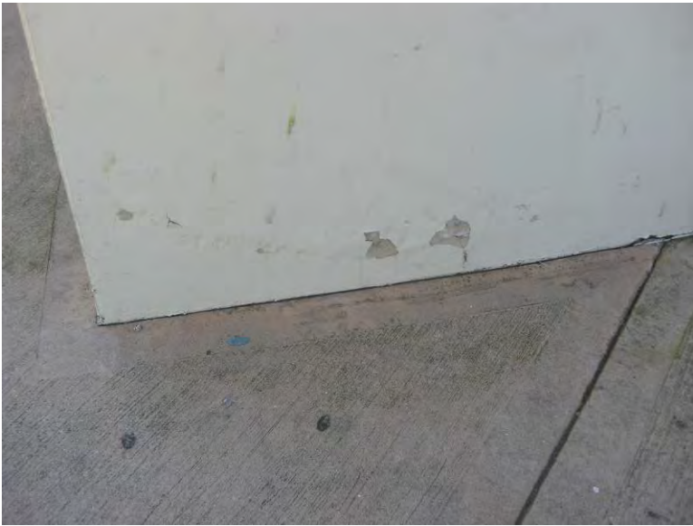
AE1. Exterior wall with paint damage.
