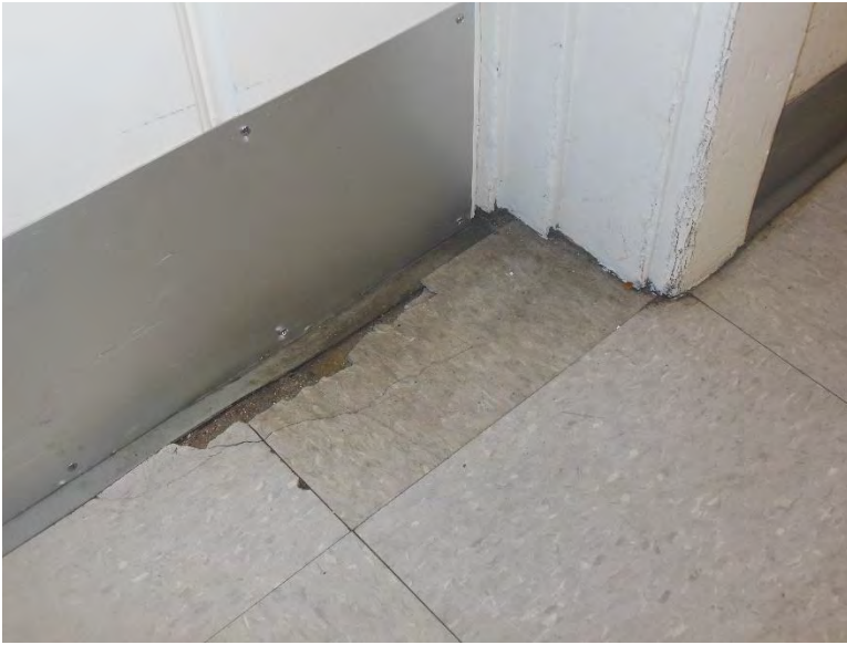
IF1. Main Office Room 8, damaged VCT at door.
