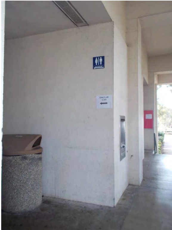
S5. Non-compliant RR signage – 2nd floor.
