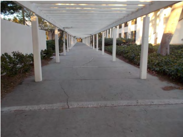
PT2. Exterior walkway Pergola; non-compliant path of travel. Concrete surface is cracked, uneven and has excessive cross slopes. ADA directional signage is not provided.
