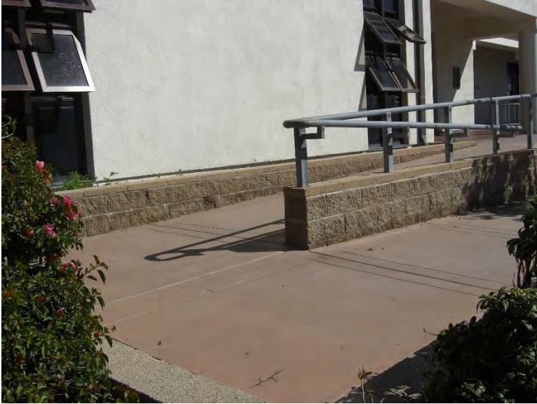
PT3. Non-compliant ramp at west main entry.
