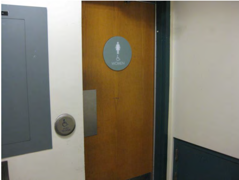
RR1. Women's Restroom; wall mounted ADA signage and electronic door opener lower-level push plate not provided.
