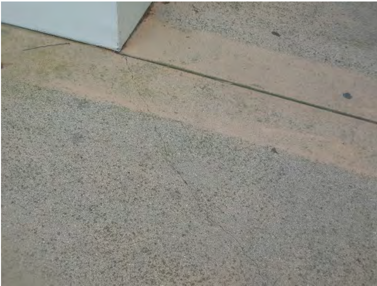
EF1. Colored concrete walkway with cracks.
