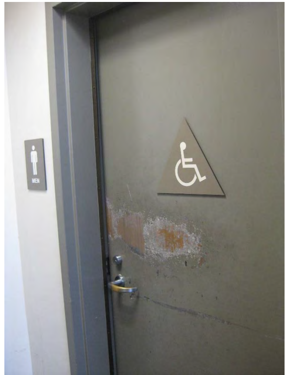
D2. Lobby Men's Restroom; damaged paint, and non-compliant door signage.
