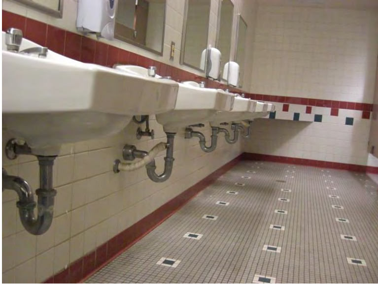
RR3. Second floor restrooms; knee protection is not provided at under sink plumbing trap.
