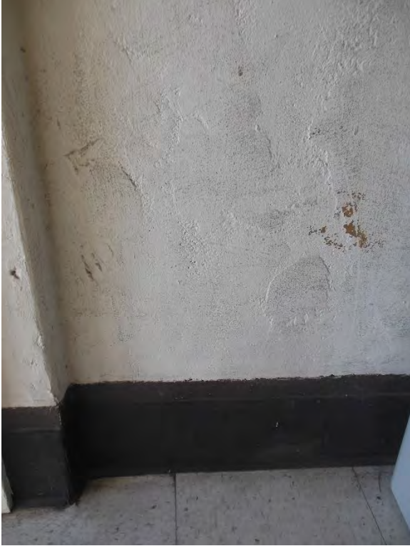
AI3. Office 11 foyer, plaster wall damage.
