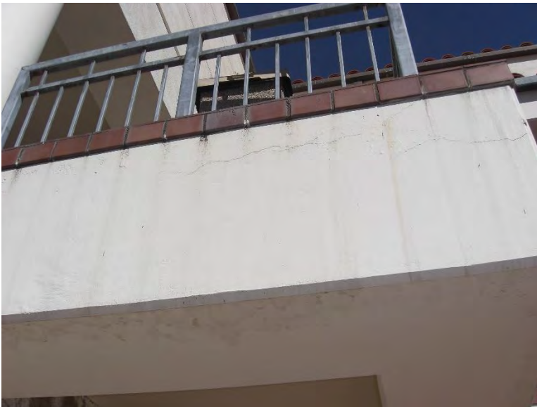
AE2. West facing entrance overhang cracked plaster finish with water damage.
