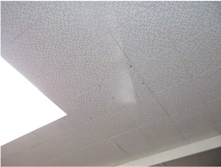
C1. Classroom; glue on ceiling tiles, typical.
