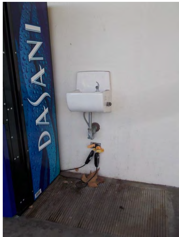
DF4. Non-compliant DF at OE first floor.
