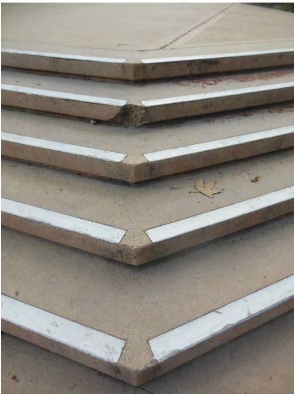
ST8. North side of building; exterior stair with damaged nosing, and missing handrail at change in stair direction.
