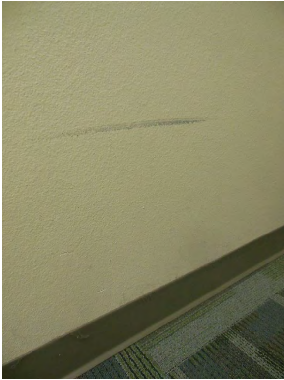
A1. Learning Center interior wall with minor damage.
