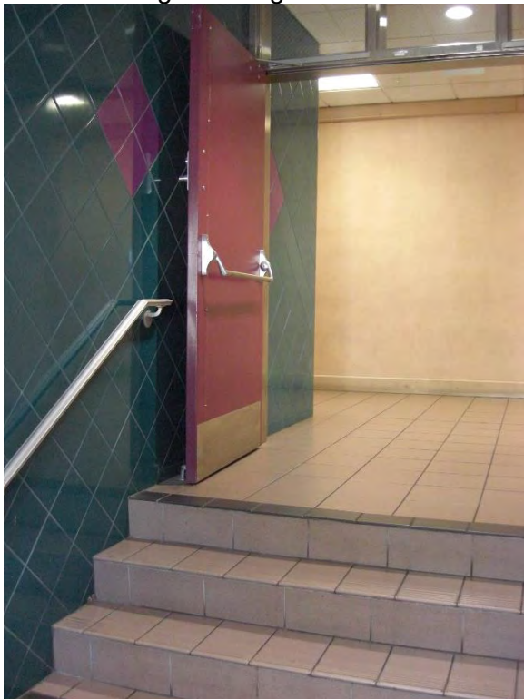
D6. Third floor, doors impede upper landing clearance.
