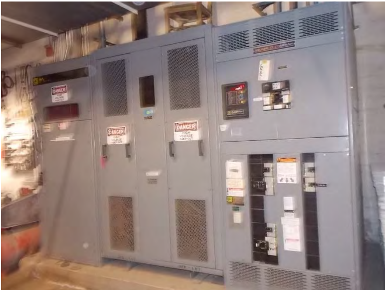
E2. Switchgear in basement.
