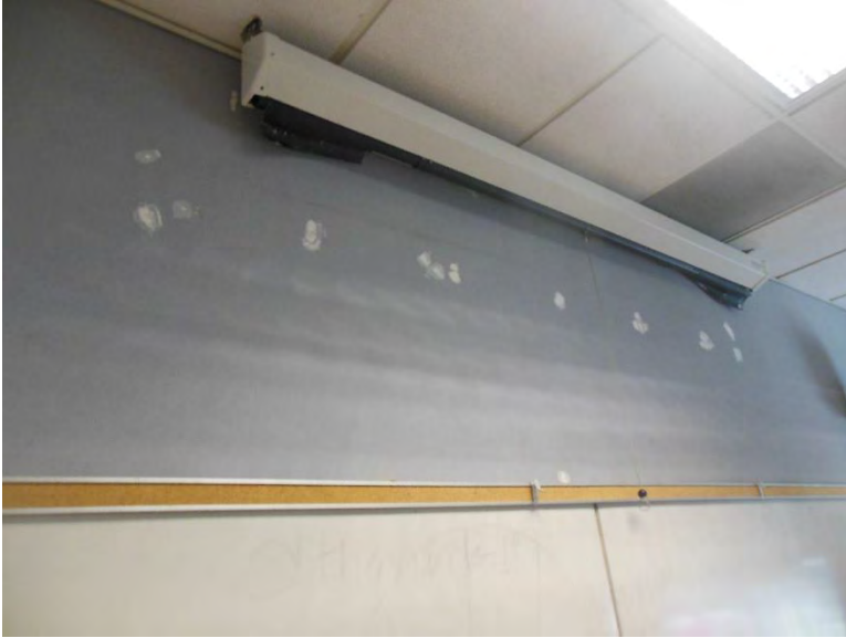
A5. Second floor classroom; wall repair damage.
