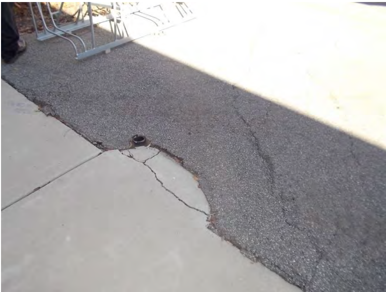
EF2. Exterior sidewalk transition; abrupt change in level.
