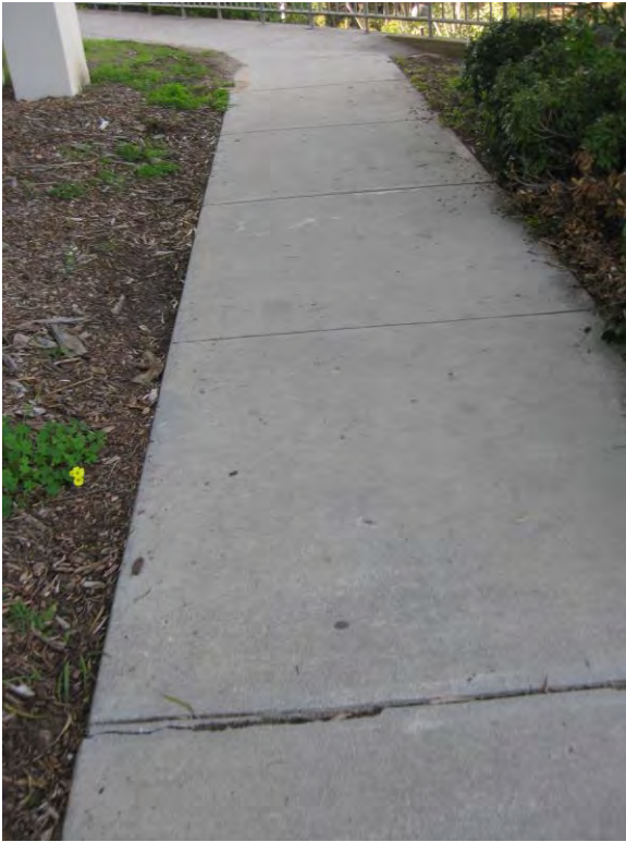
EF1. East side concrete walkway, with large cracks, tripping hazards and excessive cross slope.
