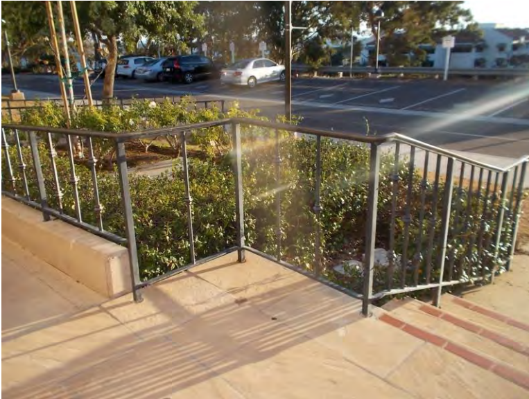
PT1. Non-compliant stairs at West main entry.
