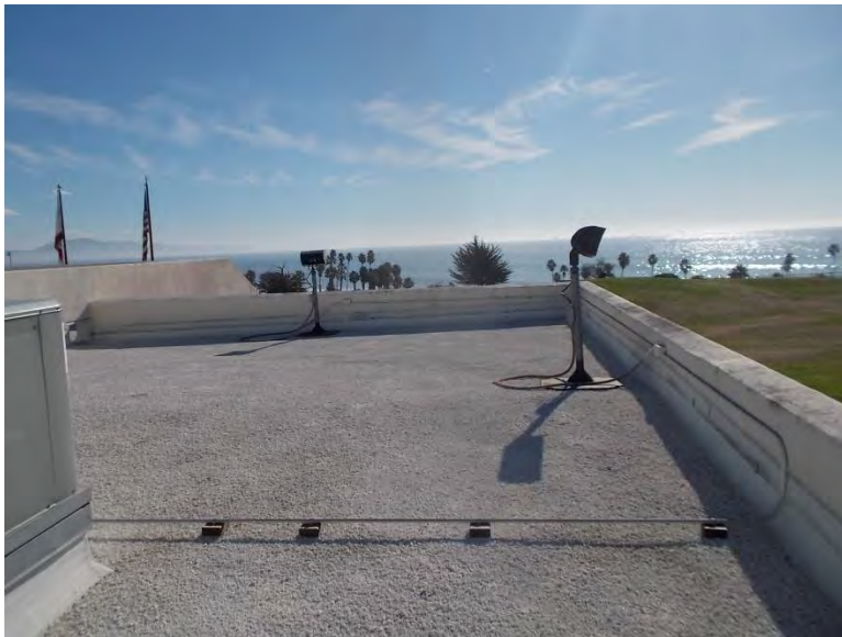
R4. Built-up roof system in good to excellent condition. Flood lights serve to light the walkways and plazas below.
