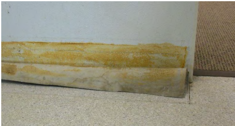
IF8. Library Café, upper floor; resilient cove base in very poor and unsanitary condition.
