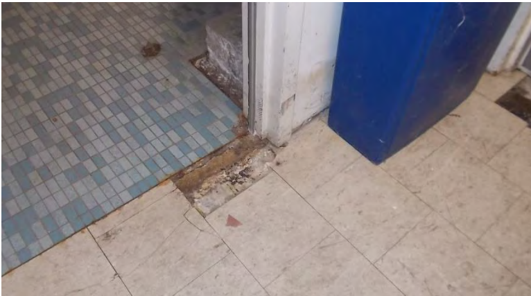
IF4. Basement; 9x9 VAT flooring damage.
