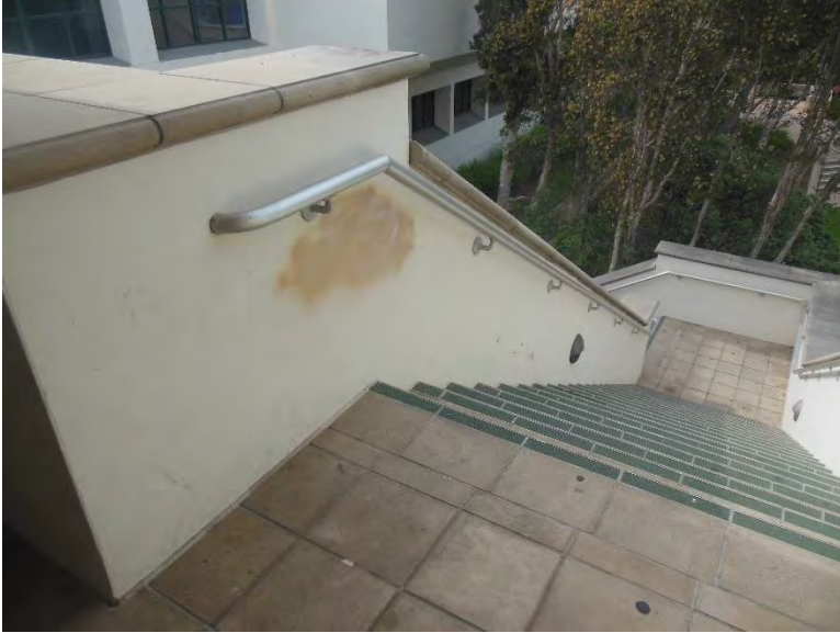
AE3. Exterior east staircase with paint damage.
