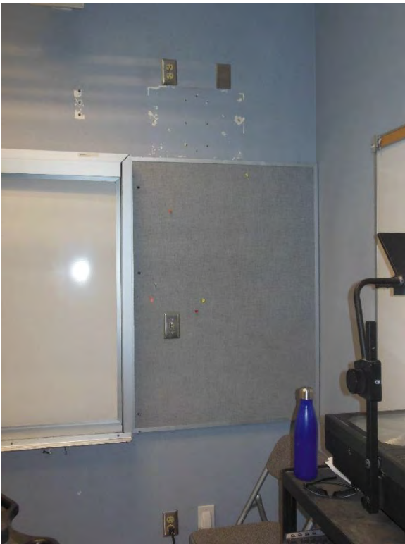
A6. Second floor classroom; wall repair damage.
