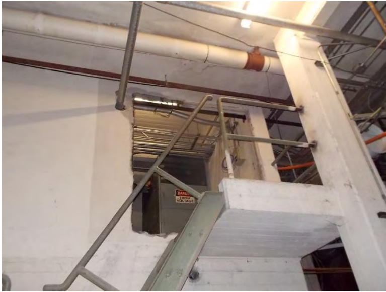
E3. Access to Electrical equipment in basement.
