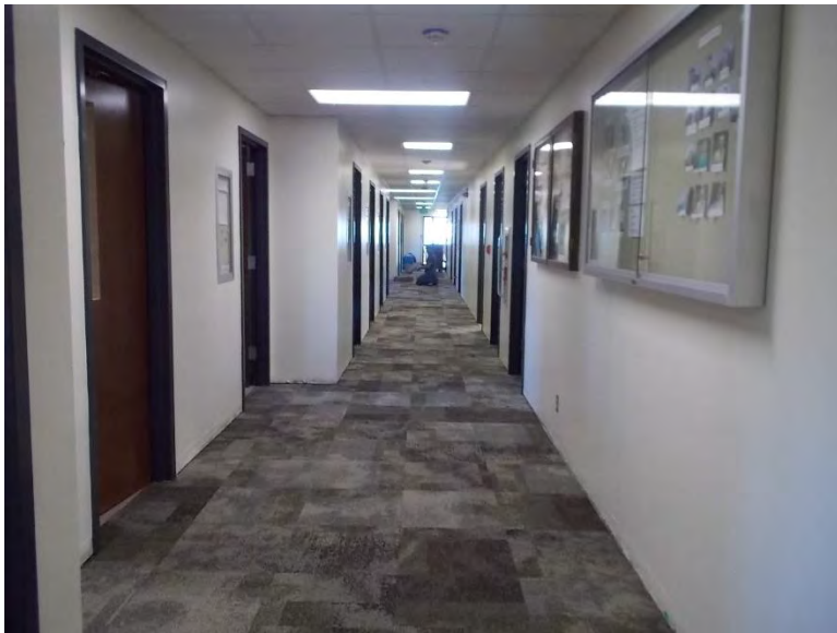
IF4. Third floor corridor carpet tile in excellent condition; installed in 2015.
