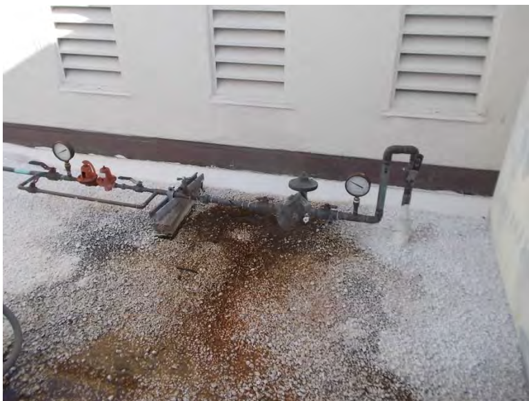
R2. Mechanical roof well with water damage at built up roofing system.
