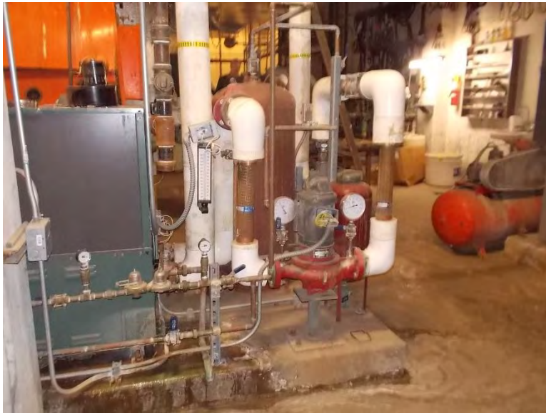
P2. Boiler piping in basement.
