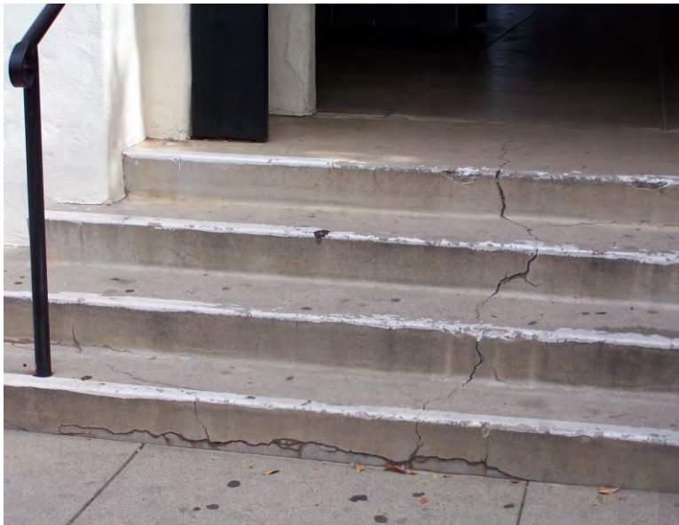
ST2. Stairs at west entrance; non-compliant handrails, stair nosing faded, and degraded concrete materials.
