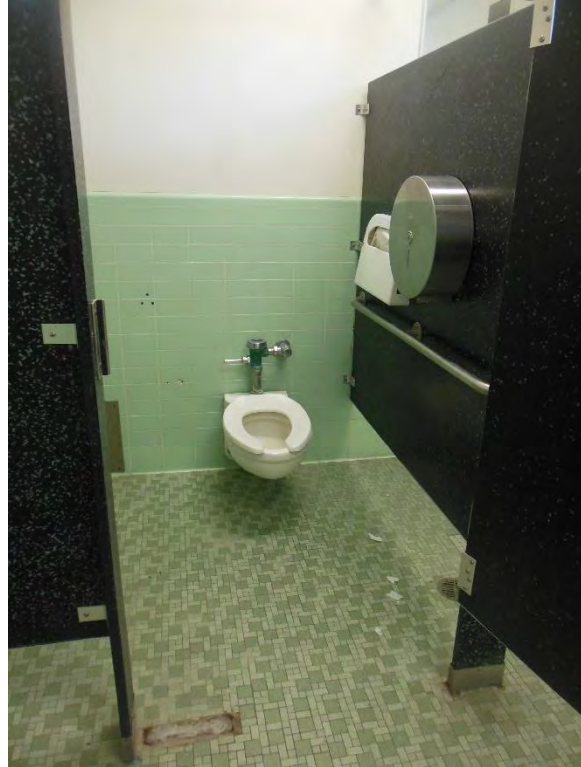
RR4. Men's Restroom; missing back handrail; and stall size too small.
