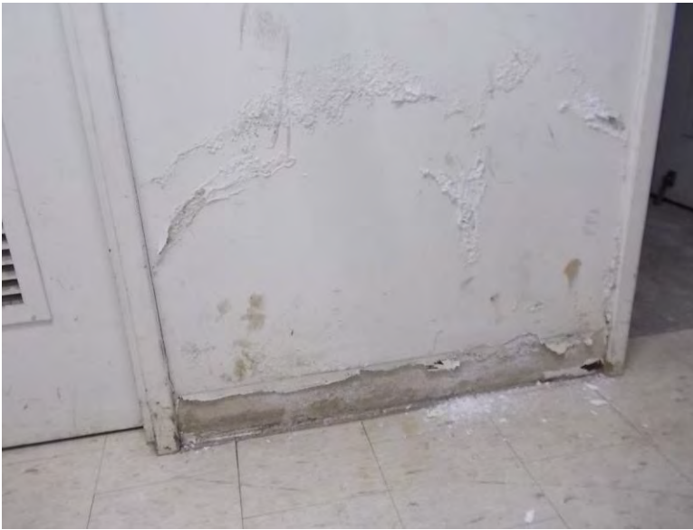
AI1. Basement; interior drywall and base damage.
