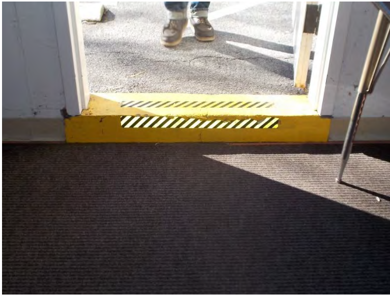
PT1. Room 32; door threshold exceeds 1/2" maximum.
