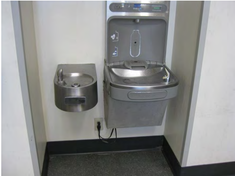
DF1. Lobby; water bottle filling station and drinking fountain.
