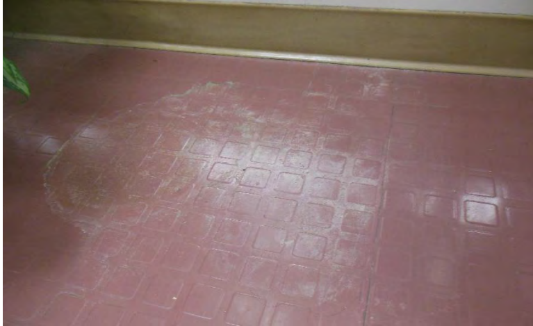
IF7. Library vestibule; rubber floor in very poor condition.
