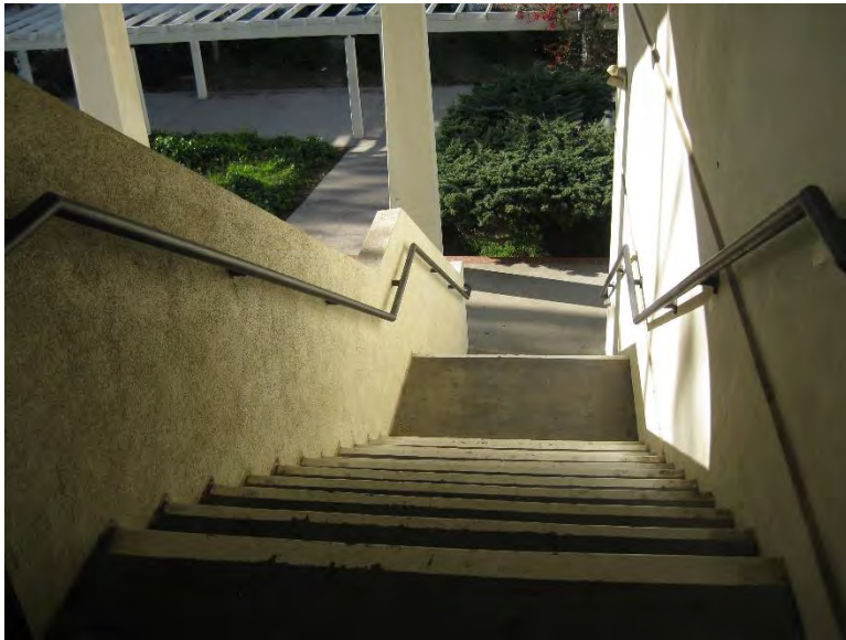
S4. Exterior northwest stair; stair nosing stripping faded, handrail heights and returns non-compliant.
