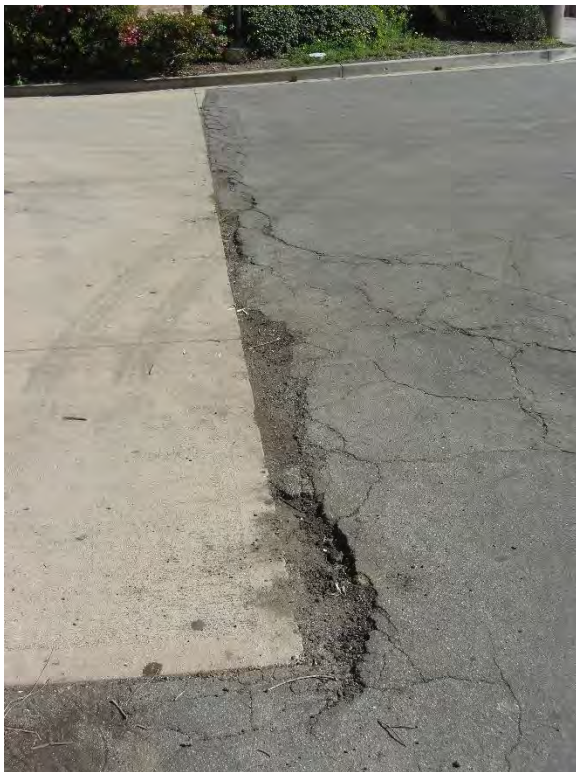
PT2. Asphalt to concrete transition along path of travel from the IDC building to the parking lot is crumbled, uneven and degraded.
