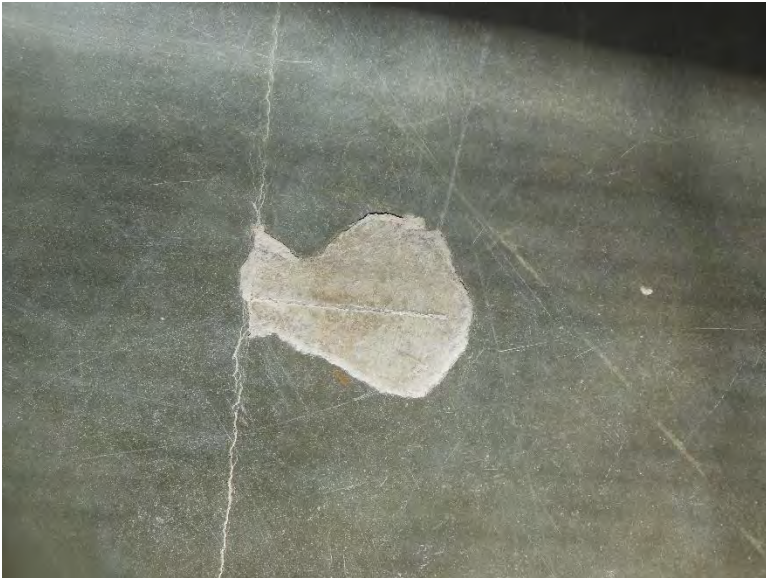
IF4. Classroom 22; concrete topping material damage.
