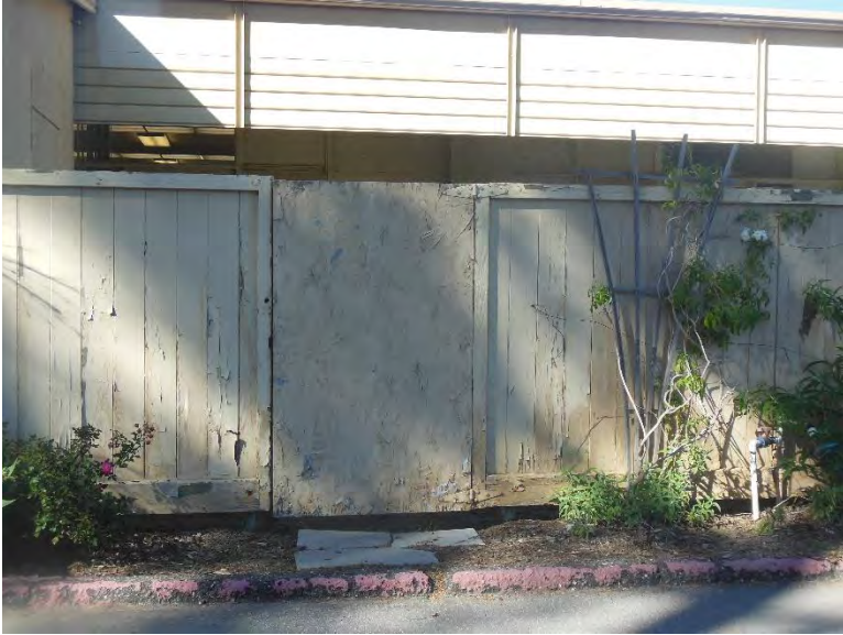
AE3. Exterior wood patio fence; damaged paint.
