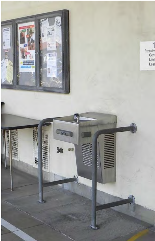
DF1. Drinking fountain in exterior walkway; hi-low fountains not provided.
