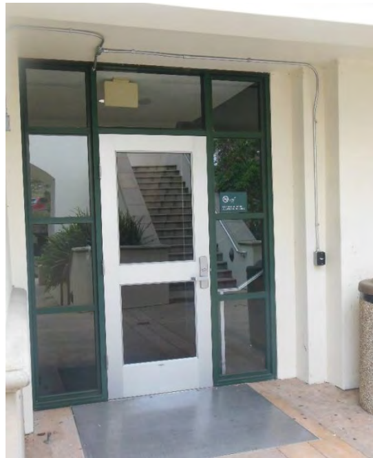
D2. Second floor entry, door lacking wall mounted room ID signage.
