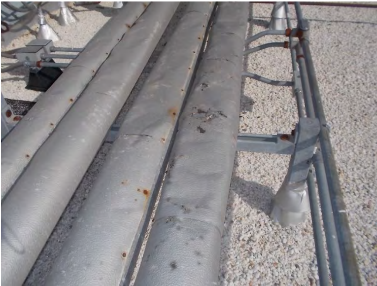
M2. Rooftop mechanical piping damaged.
