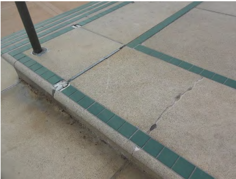
EF2. Front entry plaza stairs; concrete cracks and tile missing.
