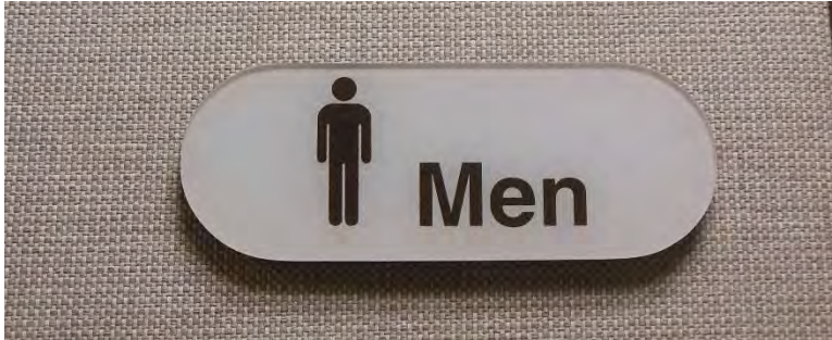
S3. Library restrooms, second floor. Women's and Men's non-compliant wall signage.
