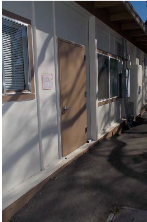
D2. Portable 22, excessive threshold height.
