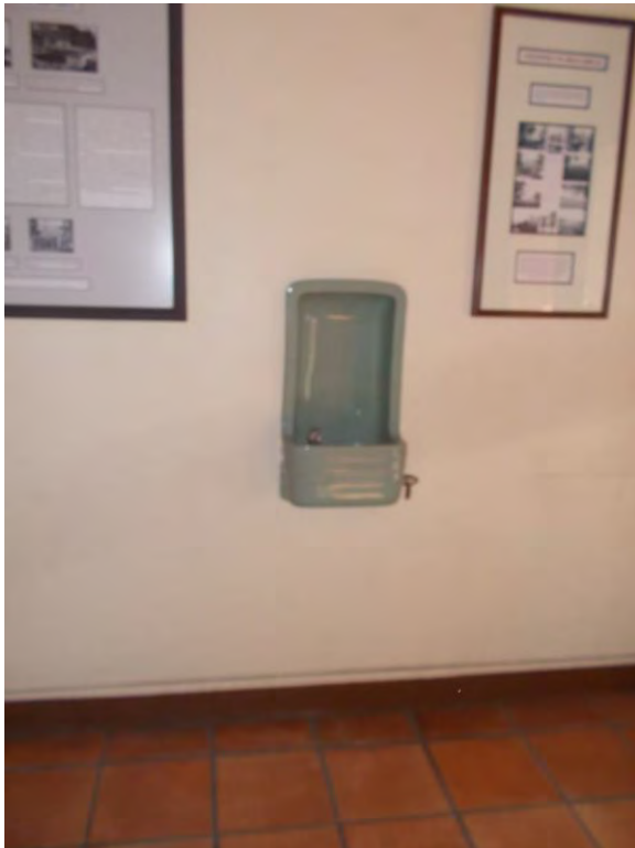
DF1. Charming era non-compliant drinking Fountain at first floor entry.
