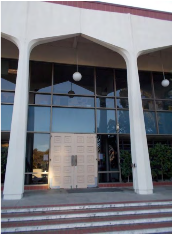
D1. East side entrance; doors require excessive force to open, electronic door opener lower-level push plate not provided and ISA sign not installed.
