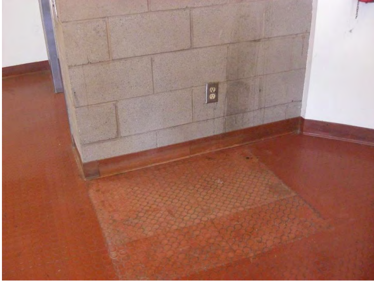
IF3. First floor exit passageway at stairwell enclosure by elevator. Damaged rubber flooring and resilient base.
