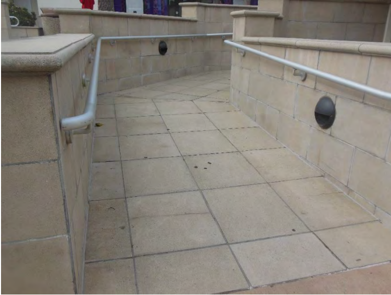
PT3. West side ramp to main building entry; intermediate landing exceeds the 2% allowed maximum cross slope.
