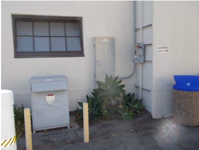
E1. Men's Restroom/Kitchen 27 exterior; electrical transformer, electrical panel and disconnect.
