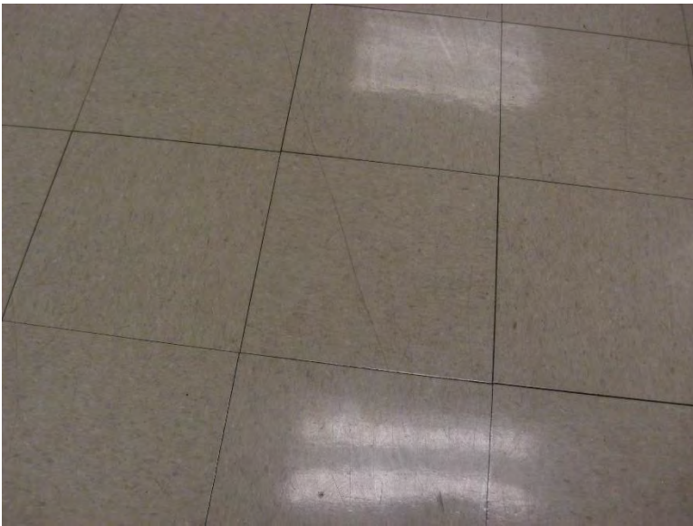
IF2. Second floor corridor; scratched/damaged VCT flooring.
