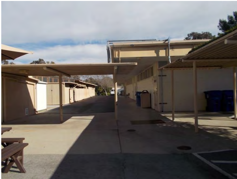
PT2. Exterior walkway; uneven, excessive slopes at path of travel.
