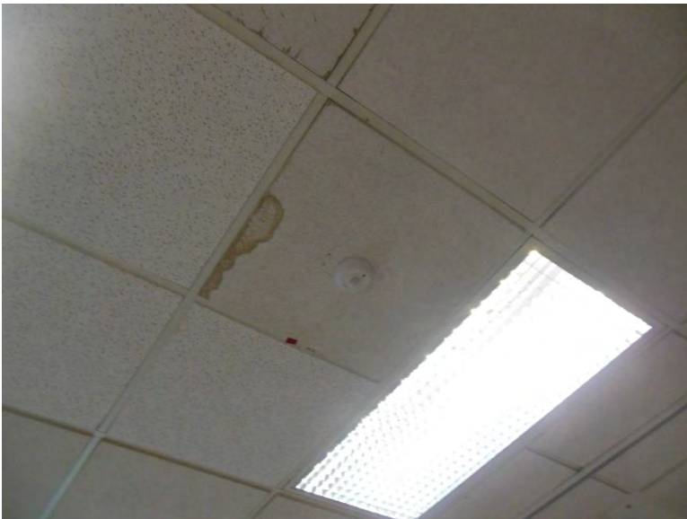
C2. Second floor classroom, stained and damaged ceiling tiles.
