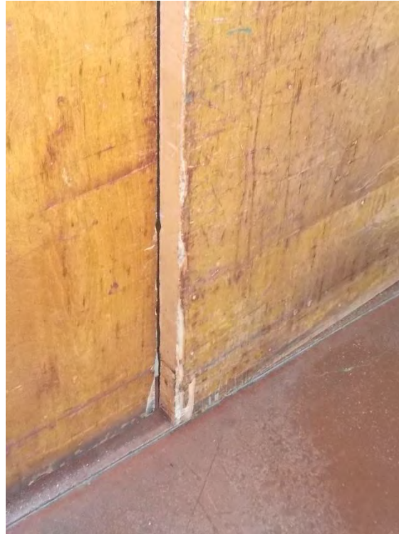
D2. Edge Damage at entrance doors.
