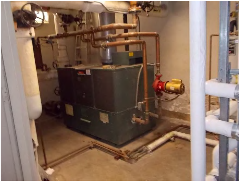
M1. Boiler in basement.
