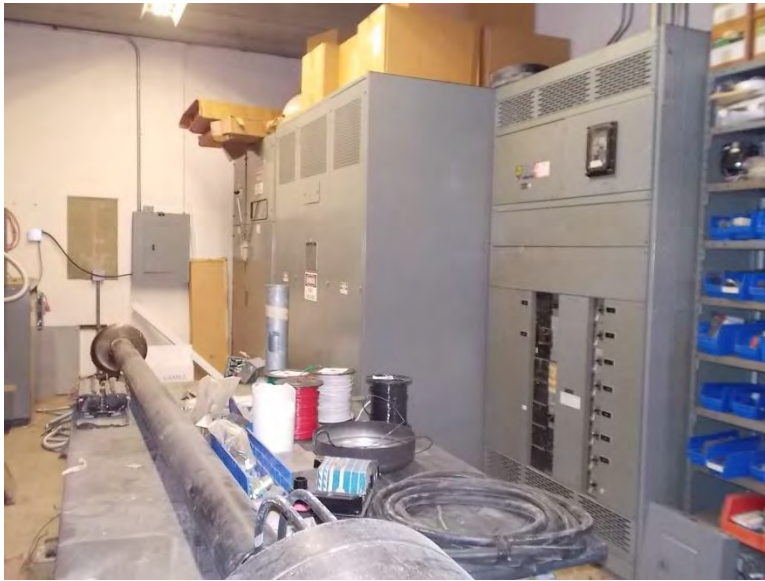
E1. Electrical equipment lacking clear floor space required by code.
