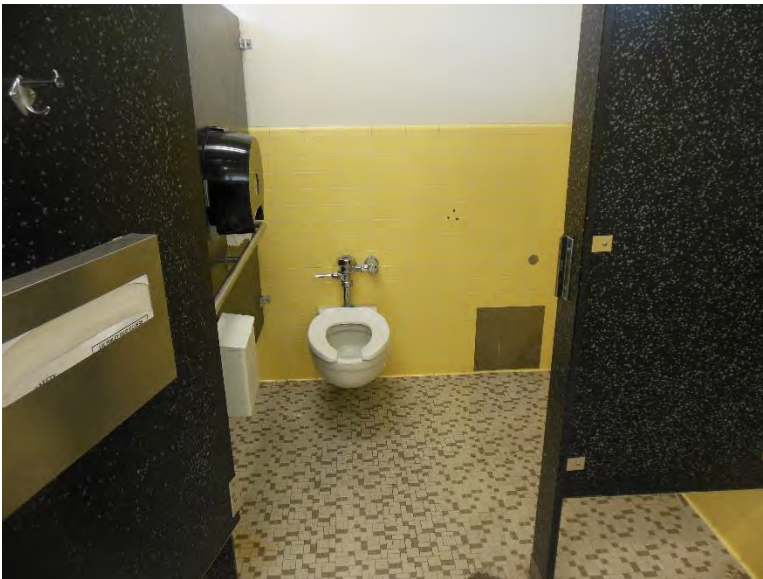
RR2. Women's Restroom; accessible stall, missing back handrail and stall size too small.
