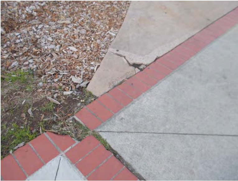
PT3. Non-compliant transition at East ramped entry.
