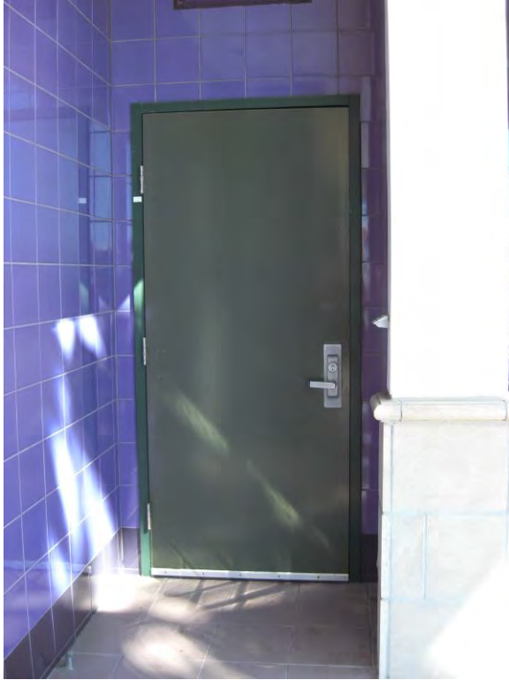
D5. Forum door; non-compliant pull-side clearance, and lacking code required door ID signage.
