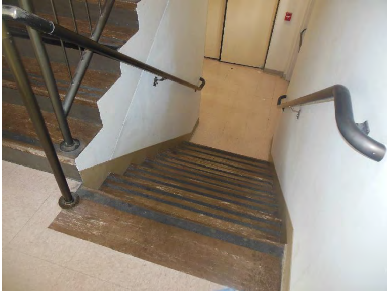
ST4. Stairwell 136; minimum stairwell width of 44" is not provided.
