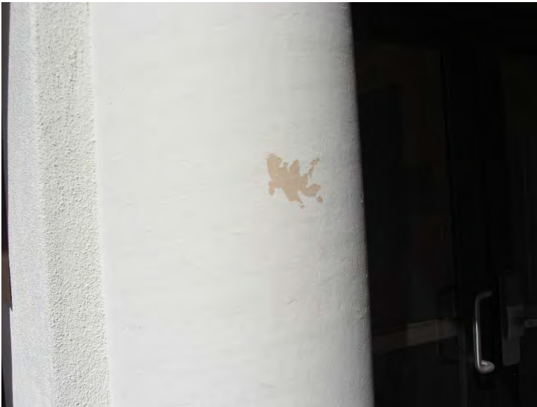
AE4. First floor CMU column under overhang with paint finish damage.
