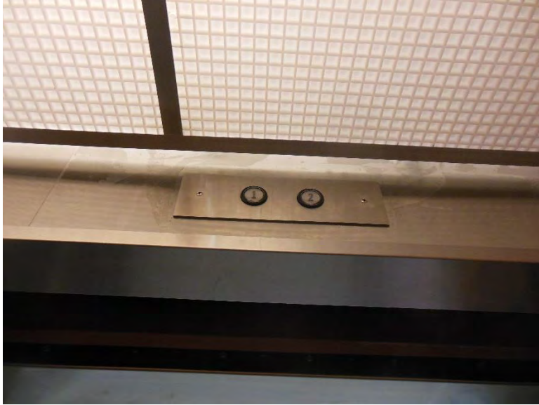
EV3. Inside elevator cab; floor indicator lights not operating.
