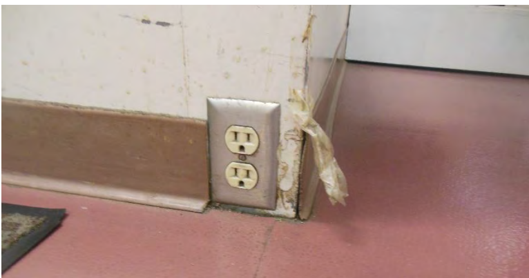
IF6. Library vestibule; resilient base in very poor condition.
