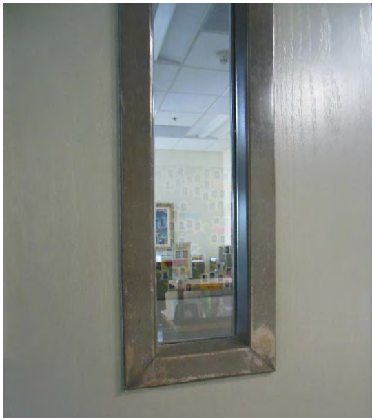
D3. Office 121; damaged frame at door lite.
