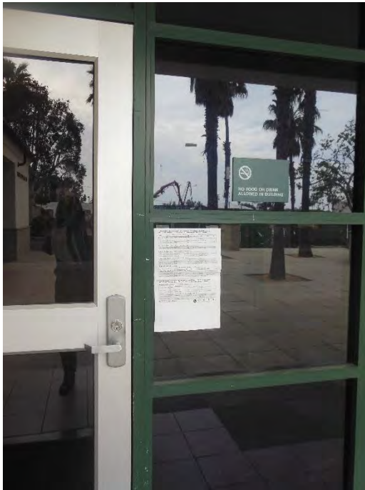
D1. Main entry; lacking wall mounted room ID signage, and an ISA symbol.
