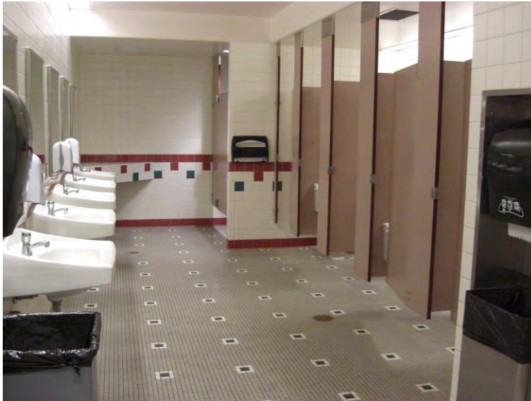
RR1. Second floor restrooms; improper placement of seat cover dispenser.
