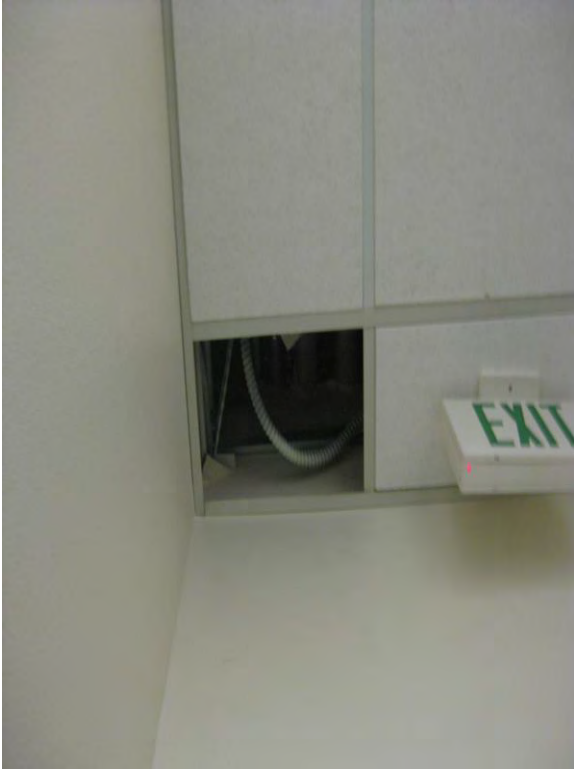
C1. Corridor 112B; missing ceiling tile.
