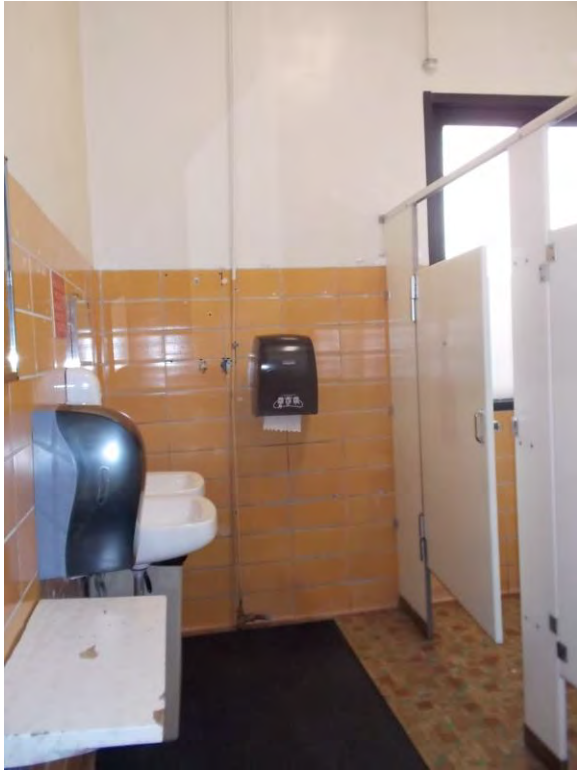
RR1. Womens non-compliant restroom, first floor northwest wing.
