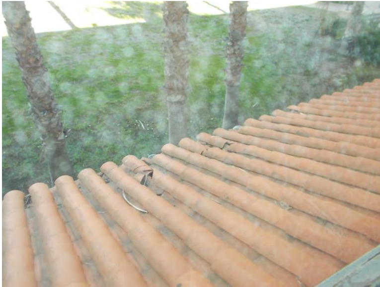
R1. Northeast roof overhang with damaged tiles.
