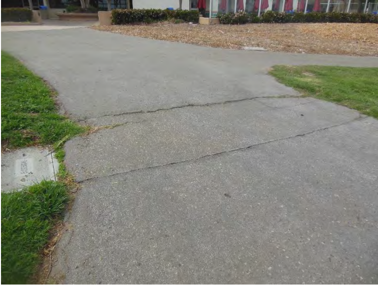
PT8. South side of building; excessive cross and longitudinal slopes, and abrupt change in level and hazardous surface features along path of travel.
