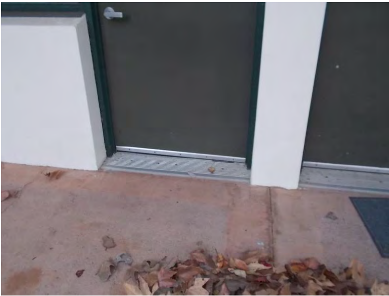
PT5. South side of building, Offices 115-117; door threshold slopes exceeds the 1/2" maximum height, and push-side dimensional clearances not provided.
