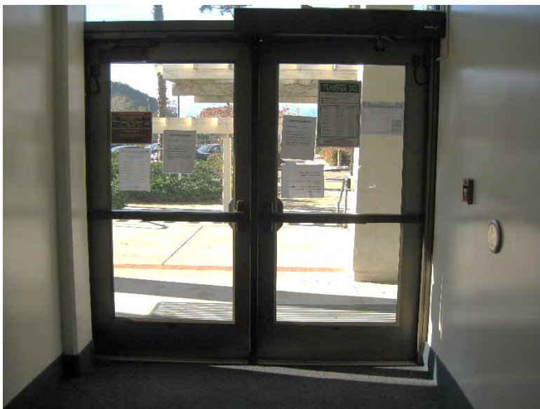
D2. First floor exit; electronic door operator low level access button required by code is not installed, and tactile exit signage not provided.
