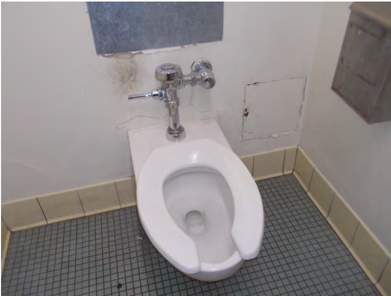
P4. Unisex –non-compliant toilet fixture, second floor northeast wing.
