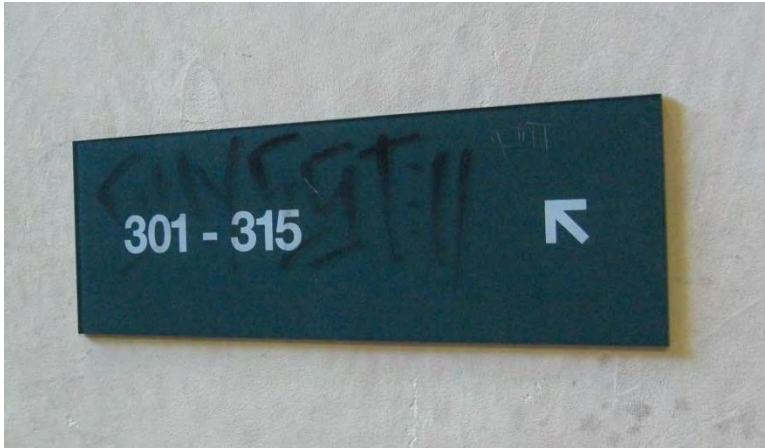
S2. Third floor; wayfinding signage vandalized.
