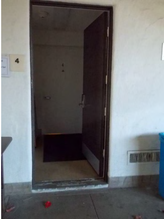
D6. Classroom 4, non-compliant threshold.
