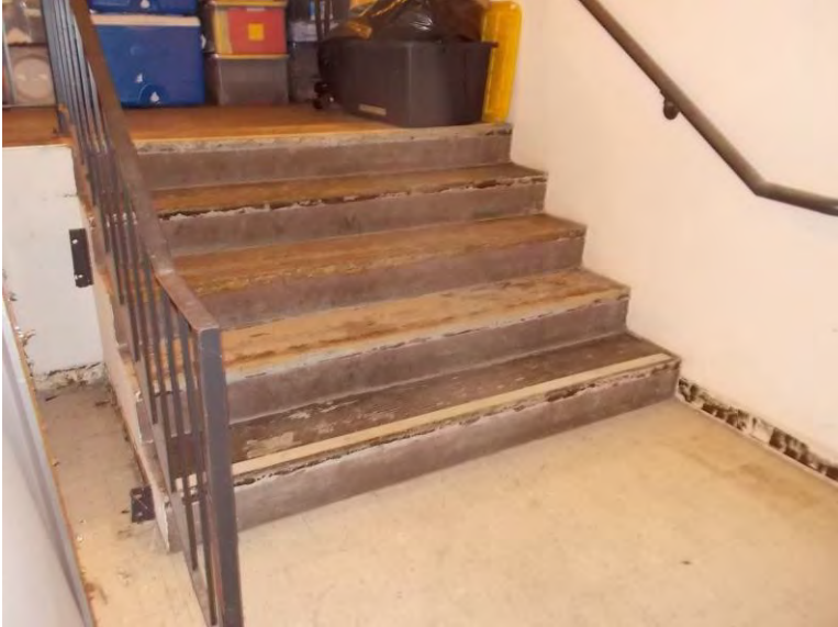
S1. Basement stairs; severely damaged materials, and non-compliant handrails.
