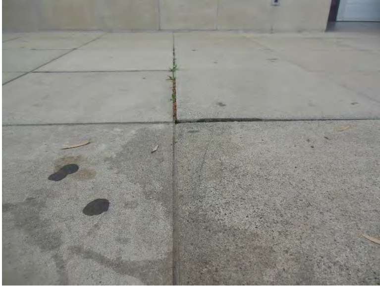
PT3. West entry plaza; abrupt change in level and hazardous surface features along path of travel.
