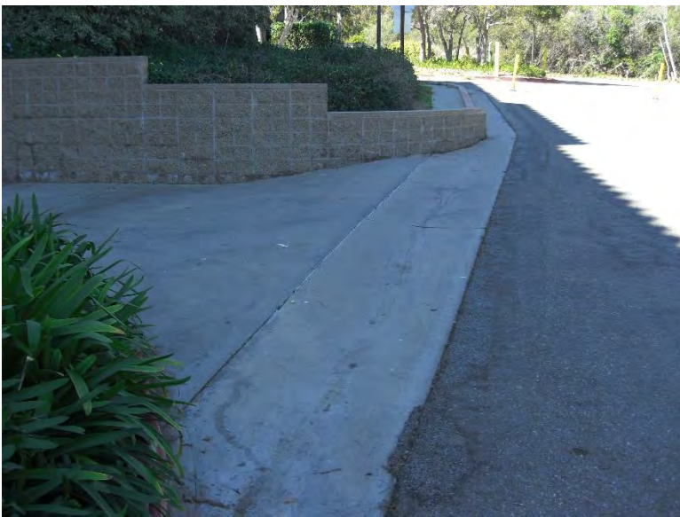
PT4. Non-compliant walkway at east main entry.
