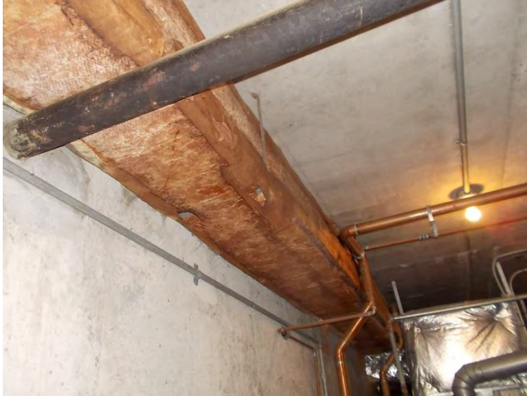
M4. Mechanical space under Kitchen; exposed insulation.
