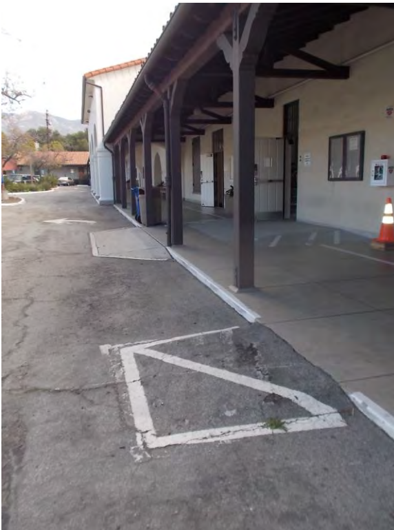
PT4. Curb ramps to parking lot; ramp cannot project into the path of cars, and are missing truncated domes. Asphalt surface is degraded.
