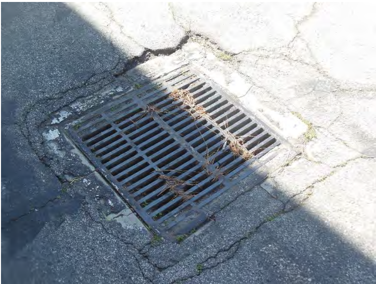
EF4. Drainage catch basin on parking lot with degraded surrounding asphalt materials.
