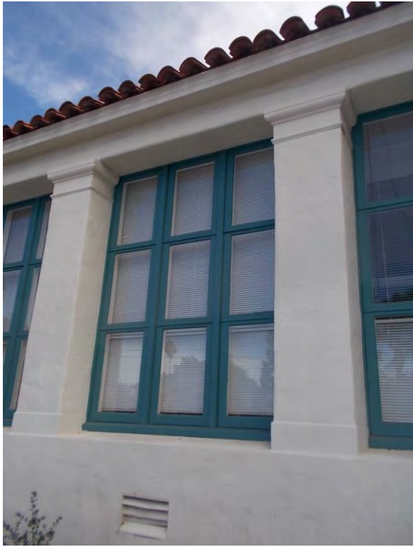
EW1. Exterior fixed wood windows; with new painted frames in excellent condition.
