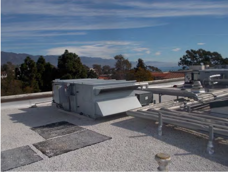
M1. Rooftop mechanical equipment.
