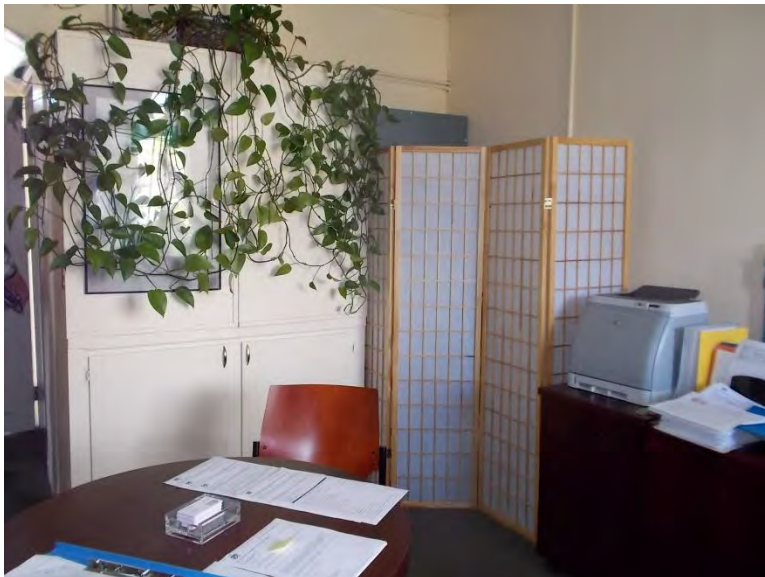
E2. Office 13 interior; main distribution panel, service meter, distribution panel and transformer, behind screen.
