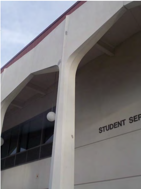
AE2. Exterior walls; peeling plaster paint.
