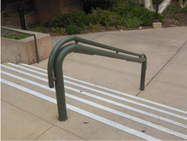
ST7. North side of building; exterior stair with non-compliant handrail heights and returns.
