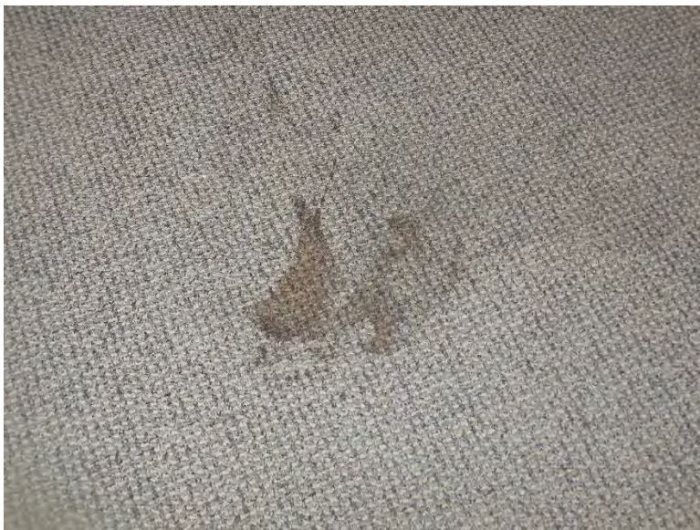
IF8. Library; broadloom carpet with stains throughout, typical.
