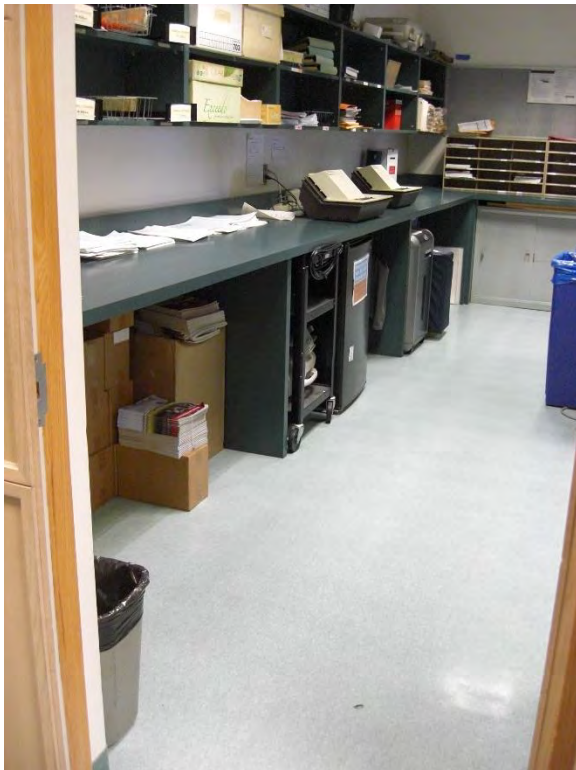
IF2. Second floor Workroom, damaged resilient floor.
