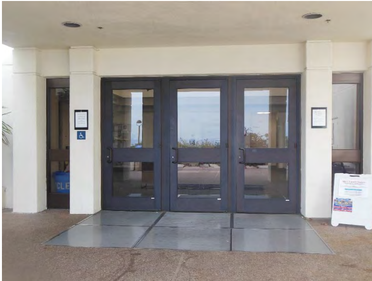
D1. Main Entrance; doors do not provide code required pull-side clearances, and wall mounted door identification signage.
