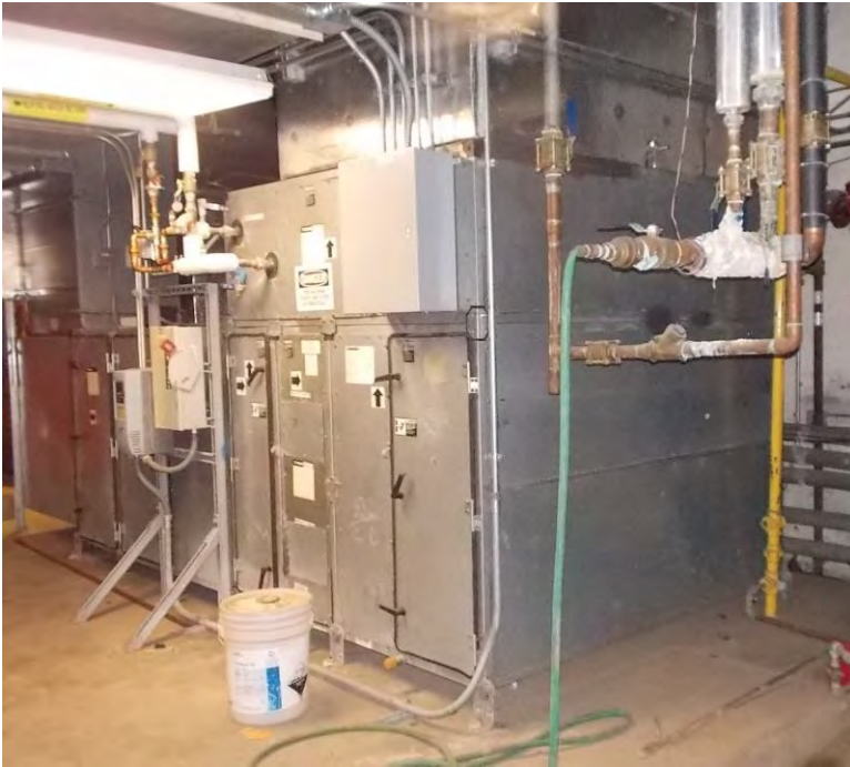
M2. AHU in basement.
