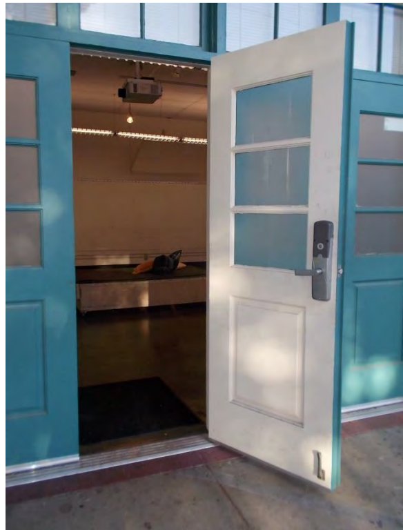
D9. Classroom 23; non-compliant thresholds and no level landing at exit.
