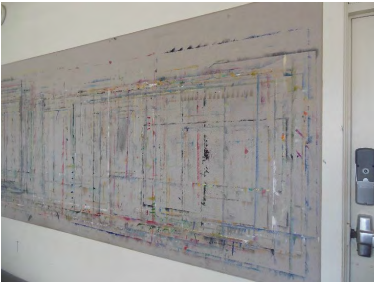
AI4. Classroom 22; fabric covered tackboard, paint damaged.
