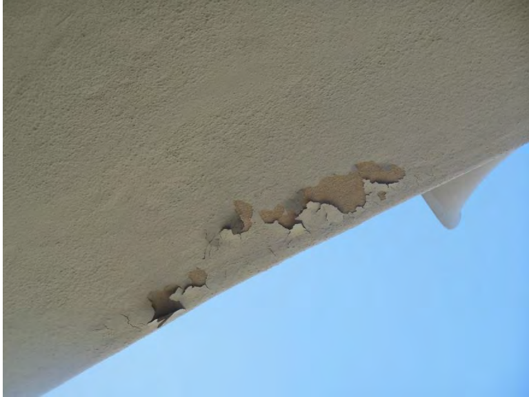
AE1. Permanent building exterior arch; peeling painted plaster.
