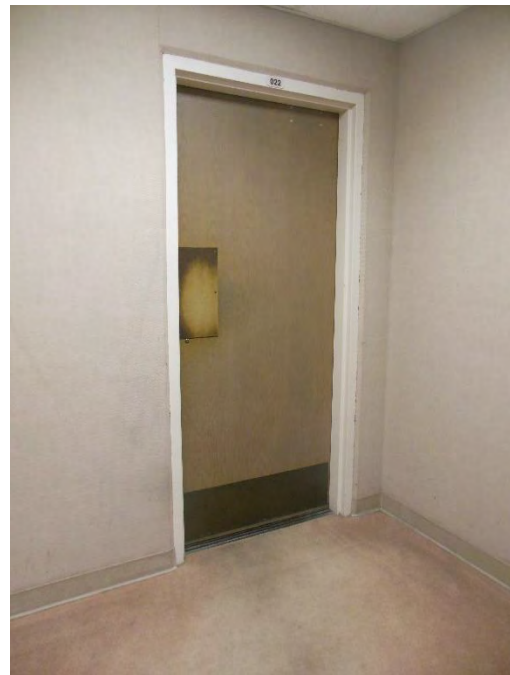
D4. Men's Restroom, 2nd floor; door and wall ADA signage not provided.
