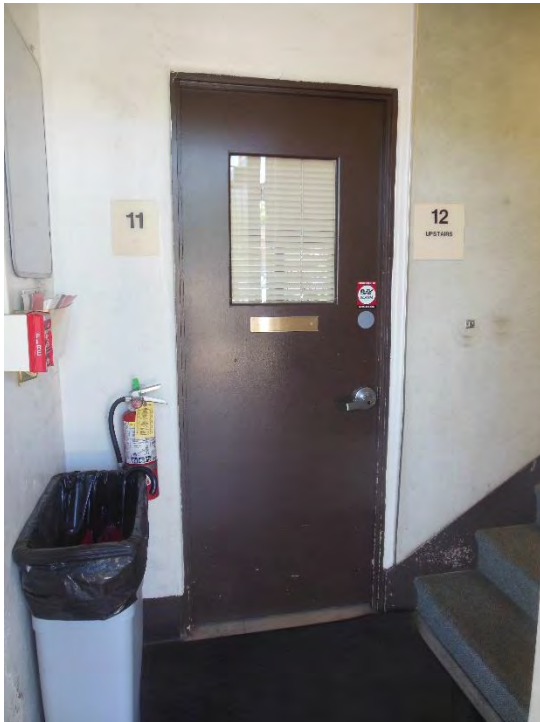
D4. Office 11; interior painted wood door; pull-side clearance not provided.
